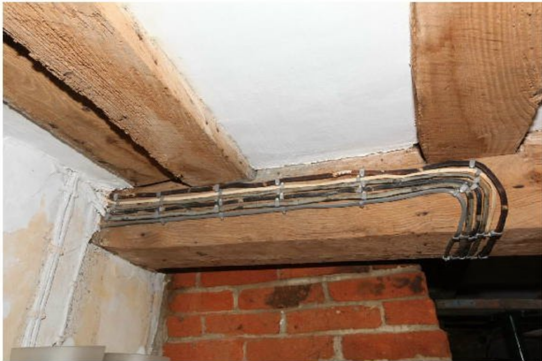
Illus. 17. A detail of the axial joist in the south-eastern bay showing the run-out chamfer stop which respects the ostensibly original chimney on the left (but not the 19 th century chimney in the centre). The joists appear to consist of elm but have been cleaned.
