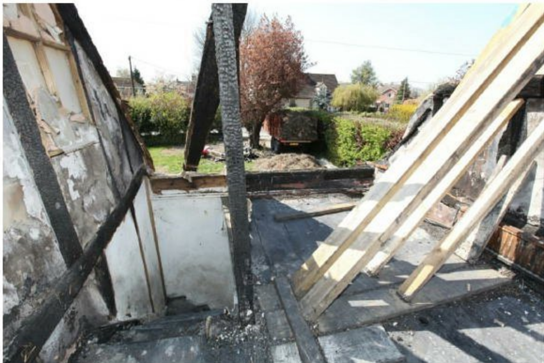
Illus. 22. The 19 th century stair landing in the service chamber looking south-west with the half-hipped gable on the right. The right-hand half of the roof-plate is original but is hidden by later boarding and has been replaced with a new oak timber on the left.
