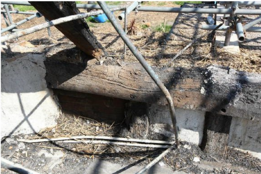
Illus. 36. A detail of the rear roof-plate in the south-eastern chamber showing a plaster-filled original dovetail joint for a missing tie-beam that formed a 1.1 m wide bay for the original chimney and corresponds with another in the front plate.
