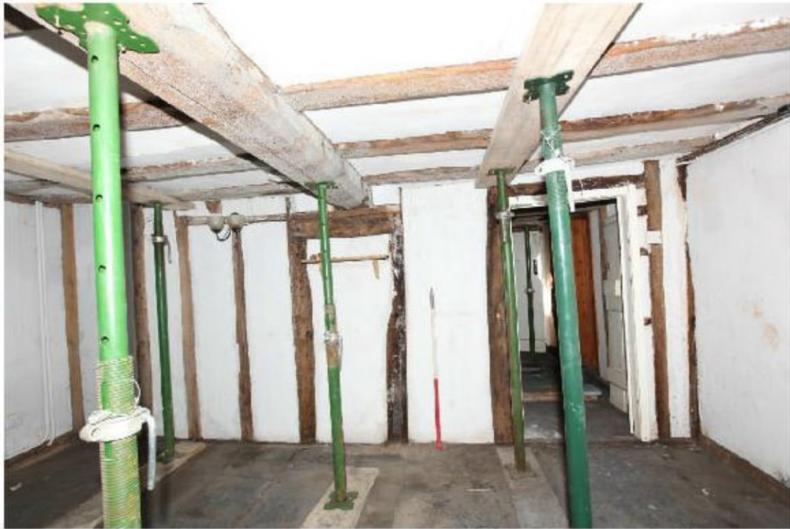
Illus. 9. The north-western wall of the central hall showing an original doorway with a pegged lintel to the right and a nailed rail supporting the axial joist of the inserted ceiling. The nailed lintel of a blocked inserted door is visible to the left of the rail but there is nothing to suggest this wall contained a second door initially.
