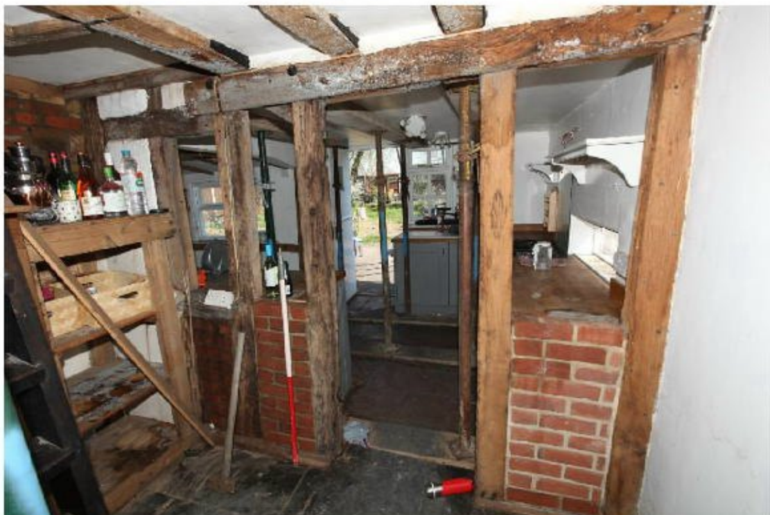
Illus. 18. The rear (north-eastern) internal wall of the parlour showing the lintel and sill of an original window on the left. This is the only section of original external wall framing exposed on the ground floor and adjoins the later lean-to containing the modern kitchen. The original ceiling joists are cut by the 19 th century chimney on the left and a modern ladder stair adjoins its brickwork.
