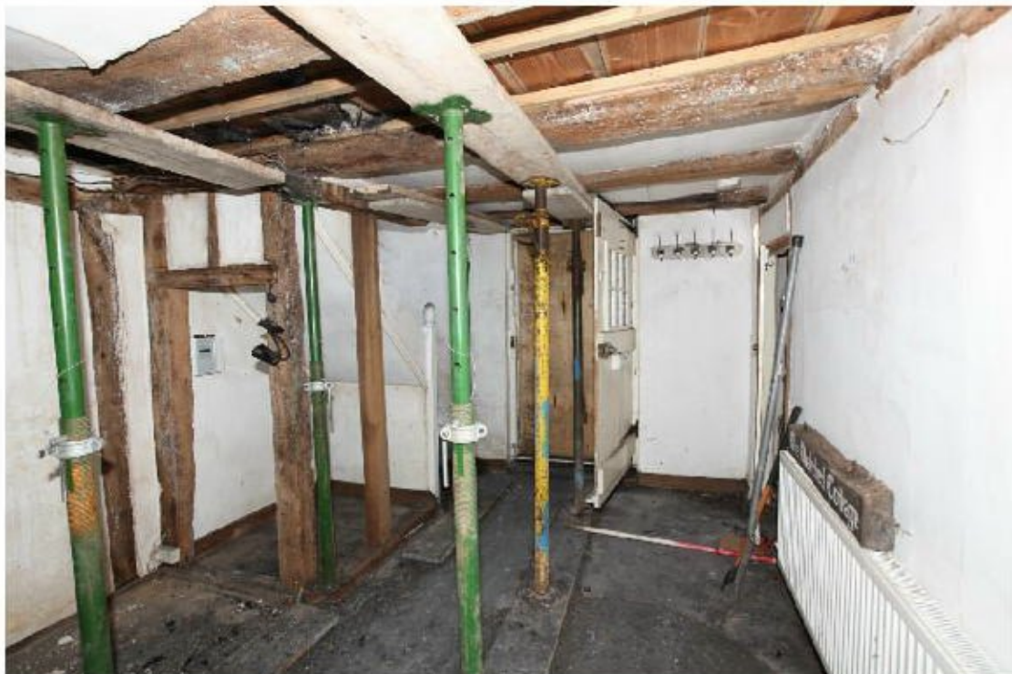
Illus. 12. The service room showing the modern entrance door in its south-western facade with the hidden fabric of the north-western gable to the right and the 19 th century staircase of pine boards to the left. The substantial ceiling joists of 18 cm by 13 (7 inches by 5) are original features lodged on pegged clamps but the vertical timbers beneath the stair are re-used 20 th century insertions.
