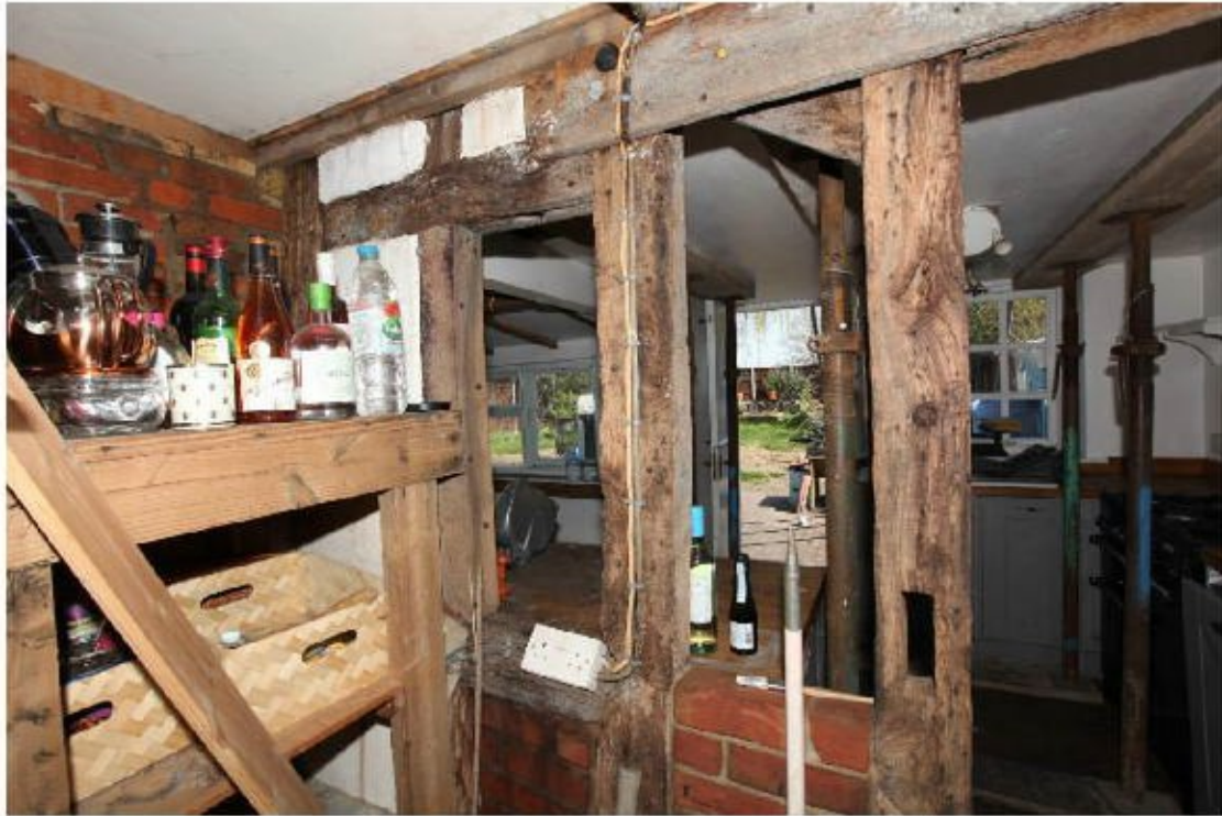
Illus. 19. The rear internal wall of the parlour with an original window lintel and sill tenoned between two studs on the left and an externally trenched brace rising from the stud on the right which is weathered internally and clearly re-used.
