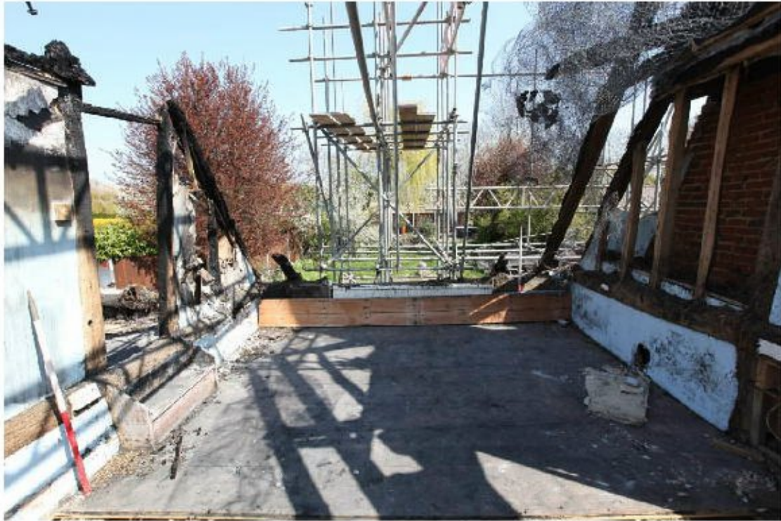
Illus. 29. The central hall chamber from the south-west showing the rear roof-plate which, like its front counterpart, has been completely renewed in modern oak.
