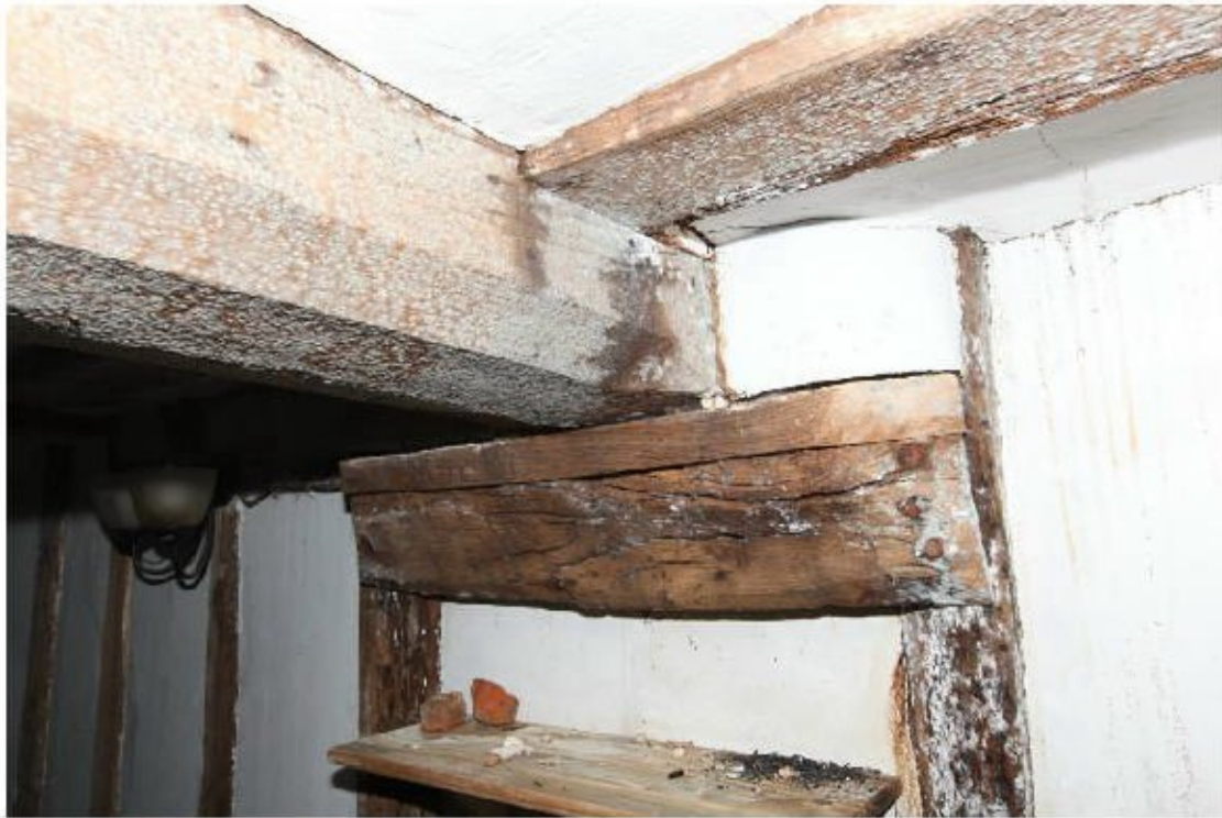
Illus. 11. A detail of the neatly chamfered axial joist of the hall ceiling supported by a short rail nailed to the original central studs of the north-western wall. This method of attachment, coupled with the lack of original first-floor doors to the hall chamber, indicates that the ceiling is a later insertion into an open hall.
