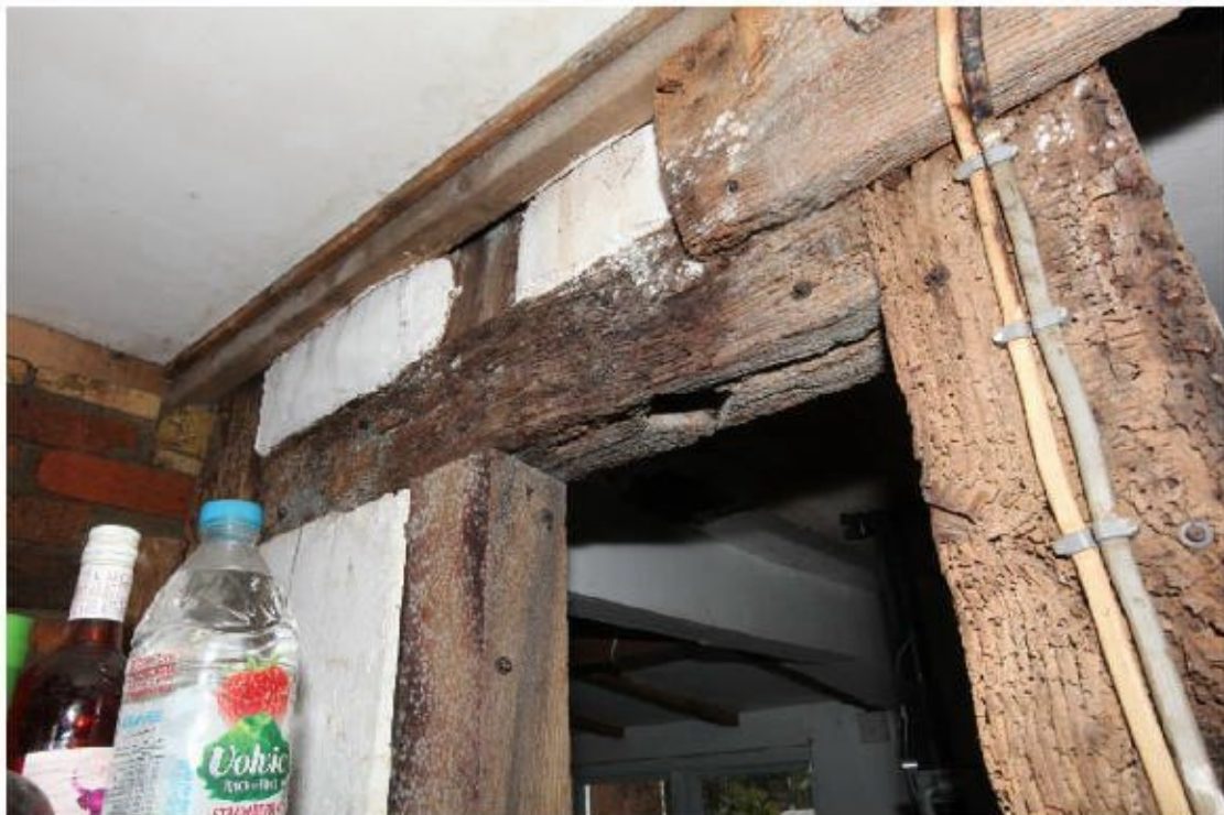
Illus. 20. A detail of the original window lintel in the rear wall of the parlour showing one of three empty mortices for diamond mullions. The nailed stud in the centre is a later insertion that blocks the window. Each mullion was 5.75 cm square (2.25 inches).
