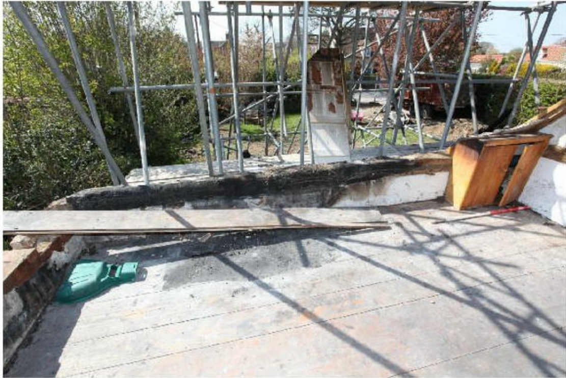
Illus. 33. The south-western roof-plate of the south-eastern bay with the gable to the left. This timber contains some pegged mortices for original studwork, albeit charred and difficult to identify, but now rests on 19 th century brickwork. A dovetail joint for a missing tie-beam that flanked the original chimney is visible to the left of the modern cupboard on the right.
