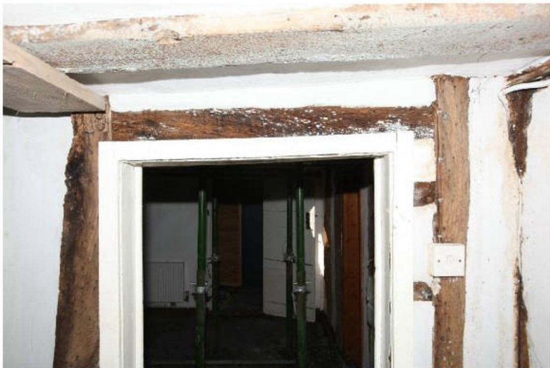
Illus. 10. A detail of the original door lintel in the north-western wall of the central hall showing the pegged joints in both jambs. The two jambs are also tenoned and pegged to the tie-beam above.
