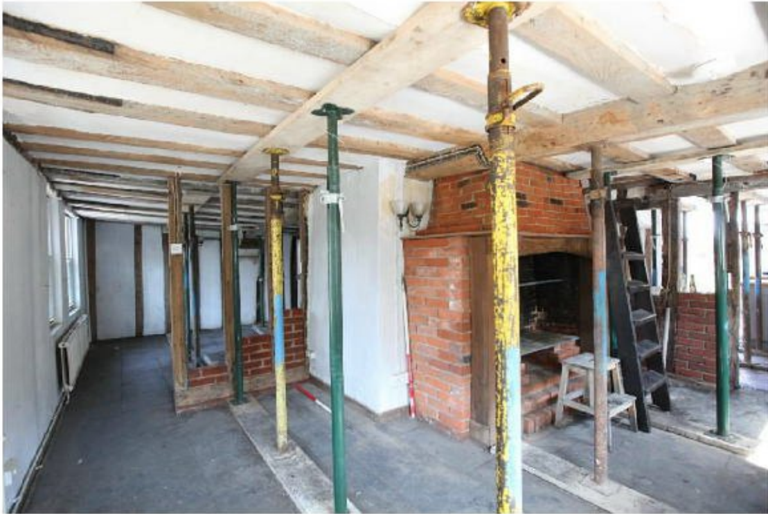
Illus. 15. The right-hand (south-eastern) bay seen from its gable with the 19 th century fireplace against the back of the rendered 16 th or 17 th century chimney in the centre. The ceiling joists adjoining the front of the earlier chimney have been renewed, suggesting that a stair may have existed here. The open studs and brickwork dividing this space from the central hall in the rear are not original.
