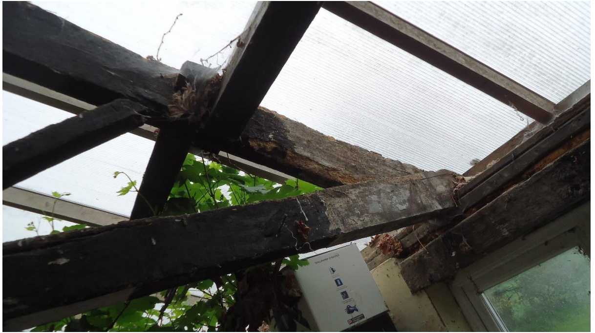
Photograph 5 Rotten roof of existing structure
