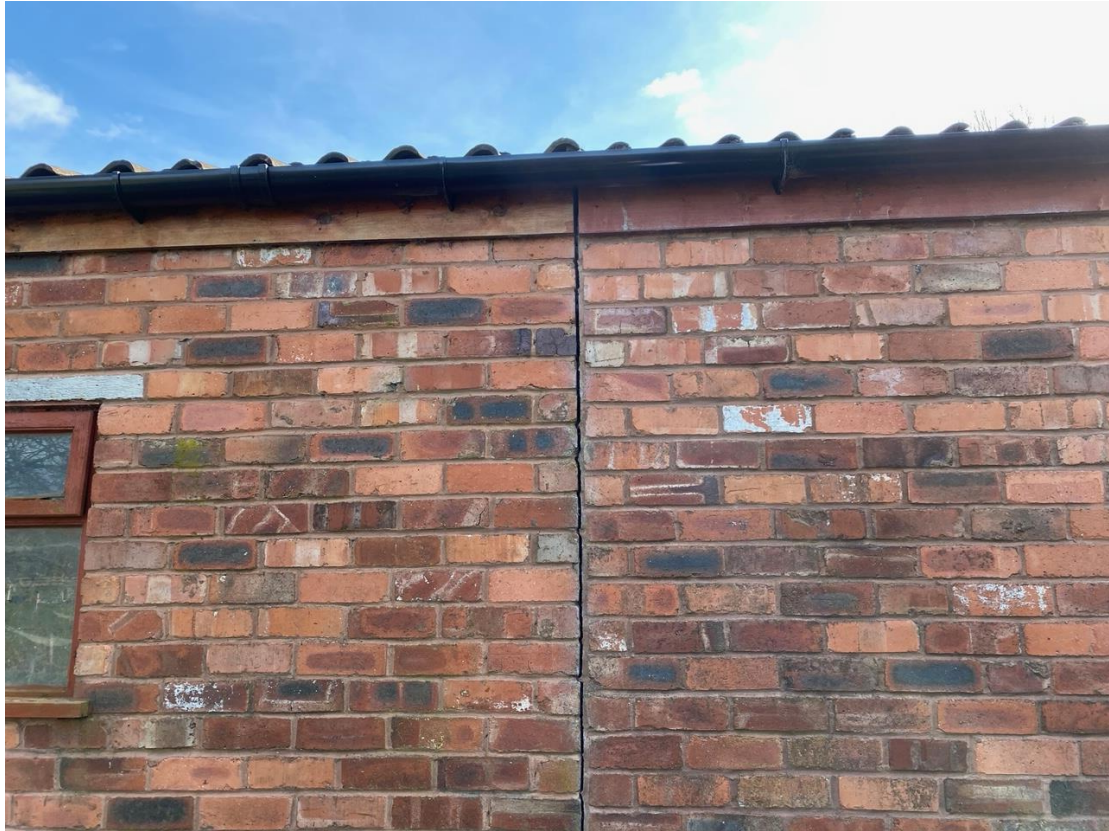
7. Vertical joint in masonry (at junction of step in floor level)
