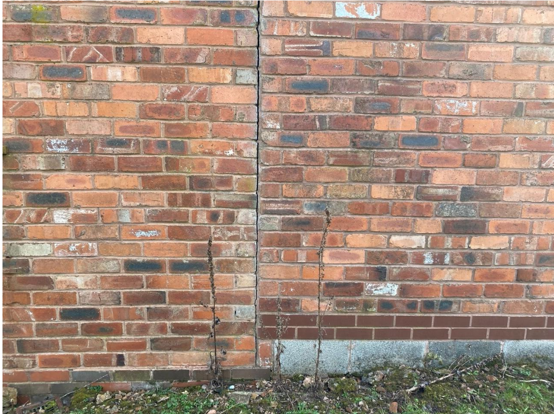
8. Vertical joint in masonry (at junction of step in floor level)
