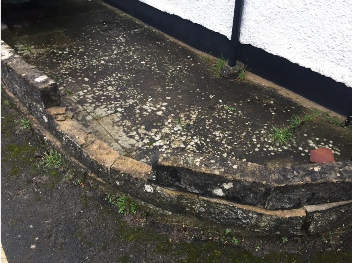
Damaged front garden wall at 9 The Croft
