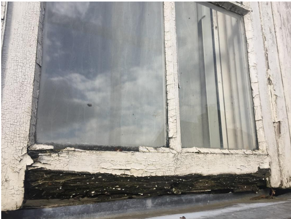
It would be possible to push a finger through the rotting wood of the middle dormer
