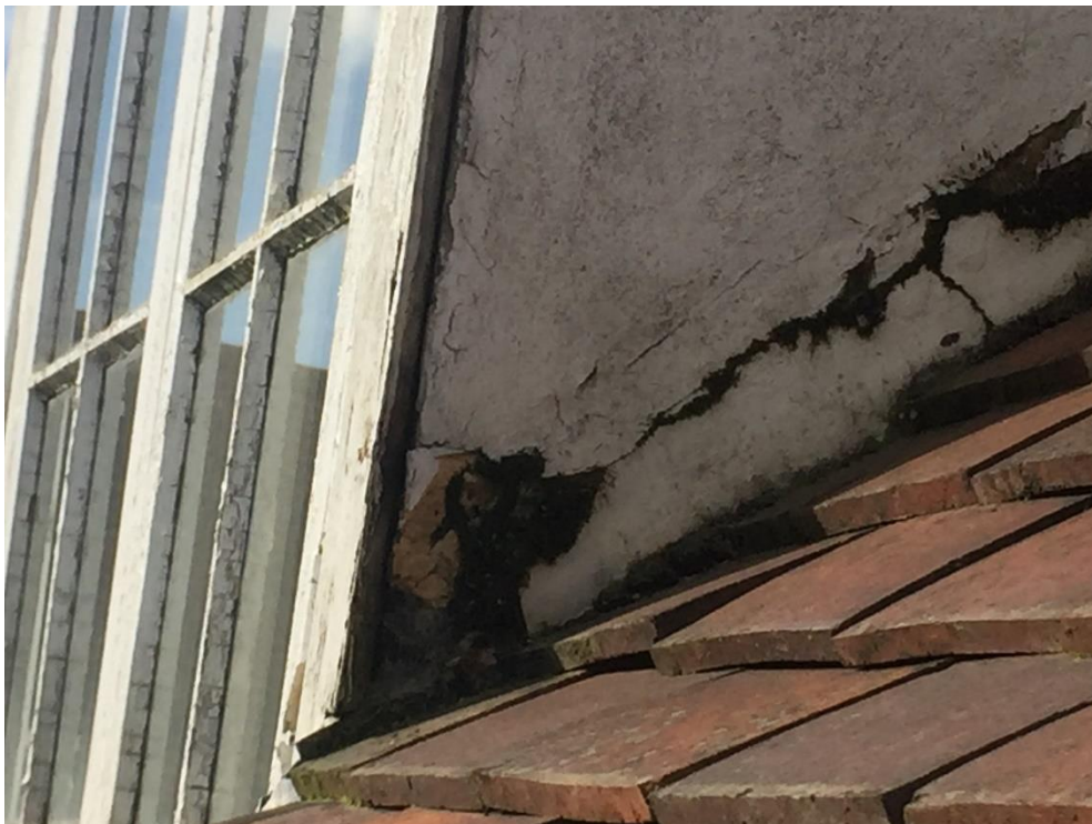
Damaged and rotting gable end
