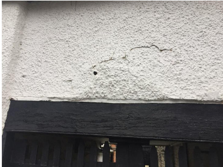
The hole and crack in the render above the gate.
