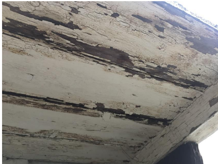
The underside of the porch cover showing the rotten wooden boards
