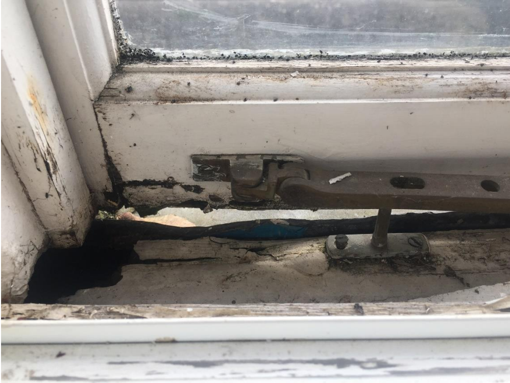
The bottom edge of the left-hand dormer casement and window have completely rotted away
