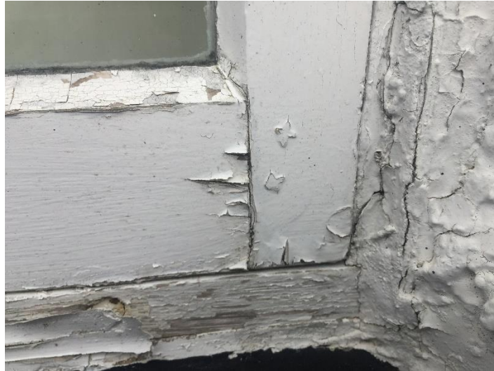
Deteriorating but relatively modern ground floor window
