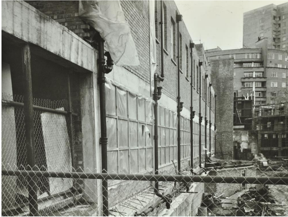
The extension to the rear of the terrace, showing reinforced concrete construction for the two storey and basement addition to the terrace. (Photo taken 1970. Source: London Metropolitan Archive)
