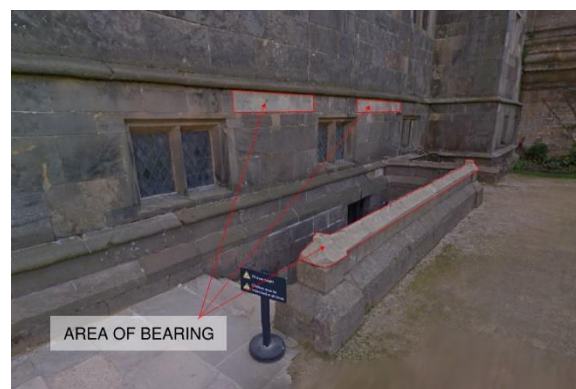
Figure 3 – Areas of bearing at external stairwell
