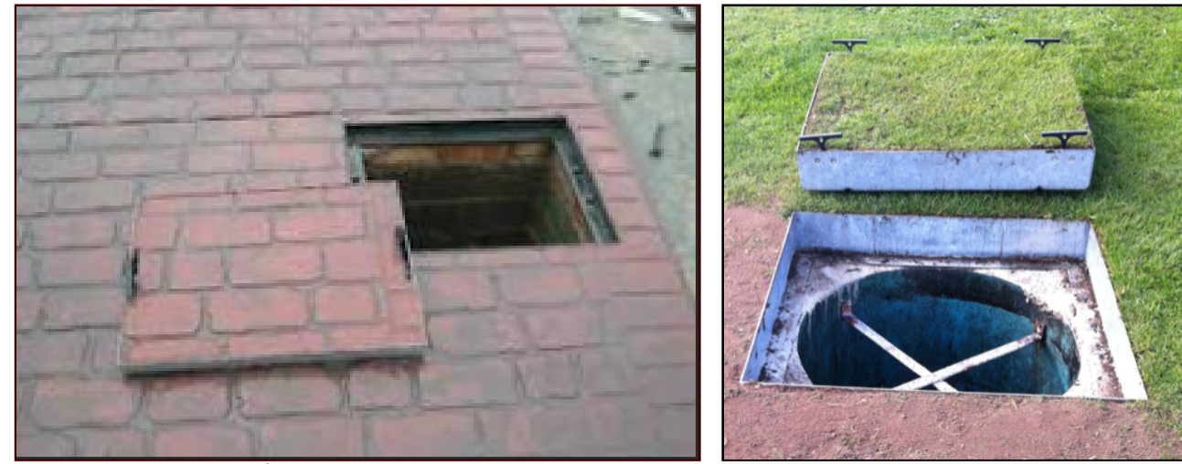
PPIC Recessed Covers to Inspection Chambers - Stone infill in to match existing stone paving in Courtyard Gavel Fill to match path material around building
