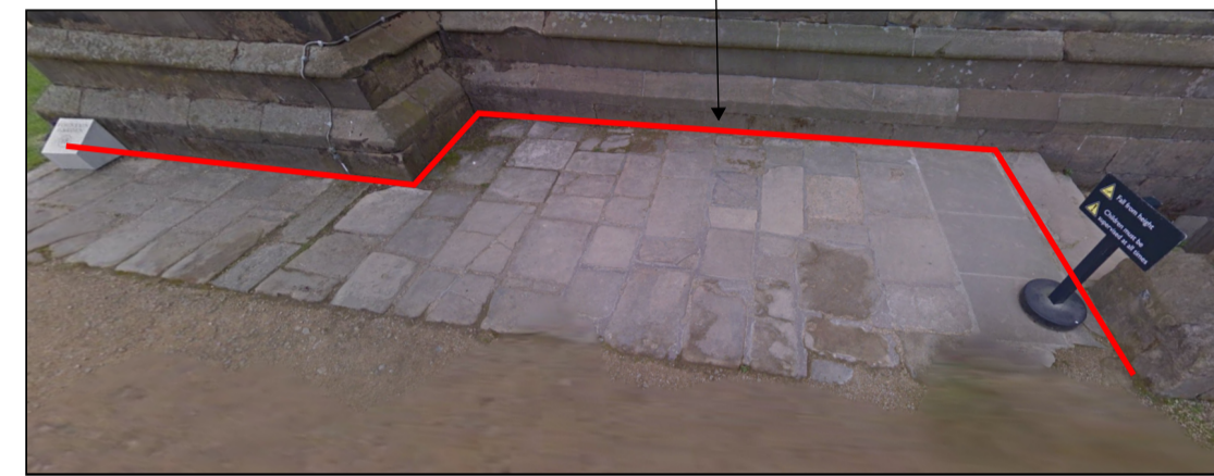
New Aco Hexdrain Brickslot installed between rear of top step and first paving flag.
