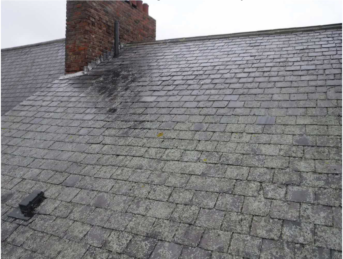
Photo 9 – Front Elevation – Roof covering between LHS chimney stack and central stack
