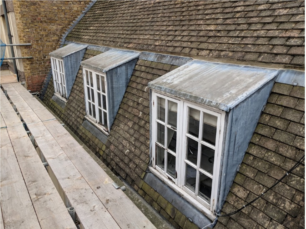
FLAT 3, 58 PETTY FRANCE WINDOWS 2021- PHOTOGRAPH BY APPLICANT 2021
