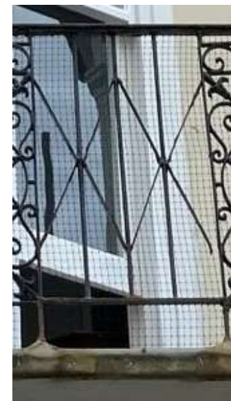
Existing inappropriate detail between larger decorative panels
