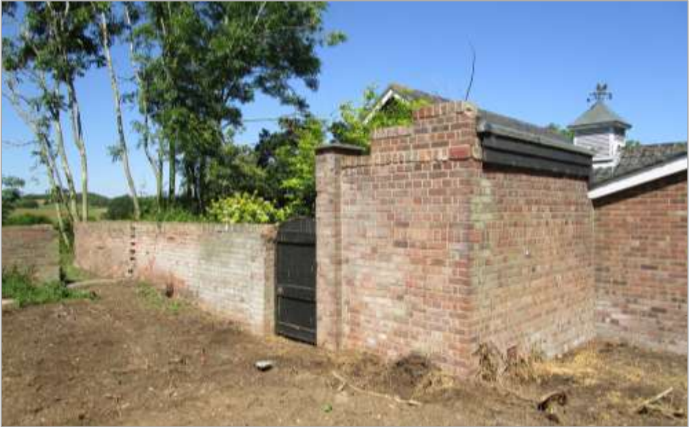
Fig.33: The courtyard from the SW, with wall largely rebuilt in Flettons following removal of nearby structures
