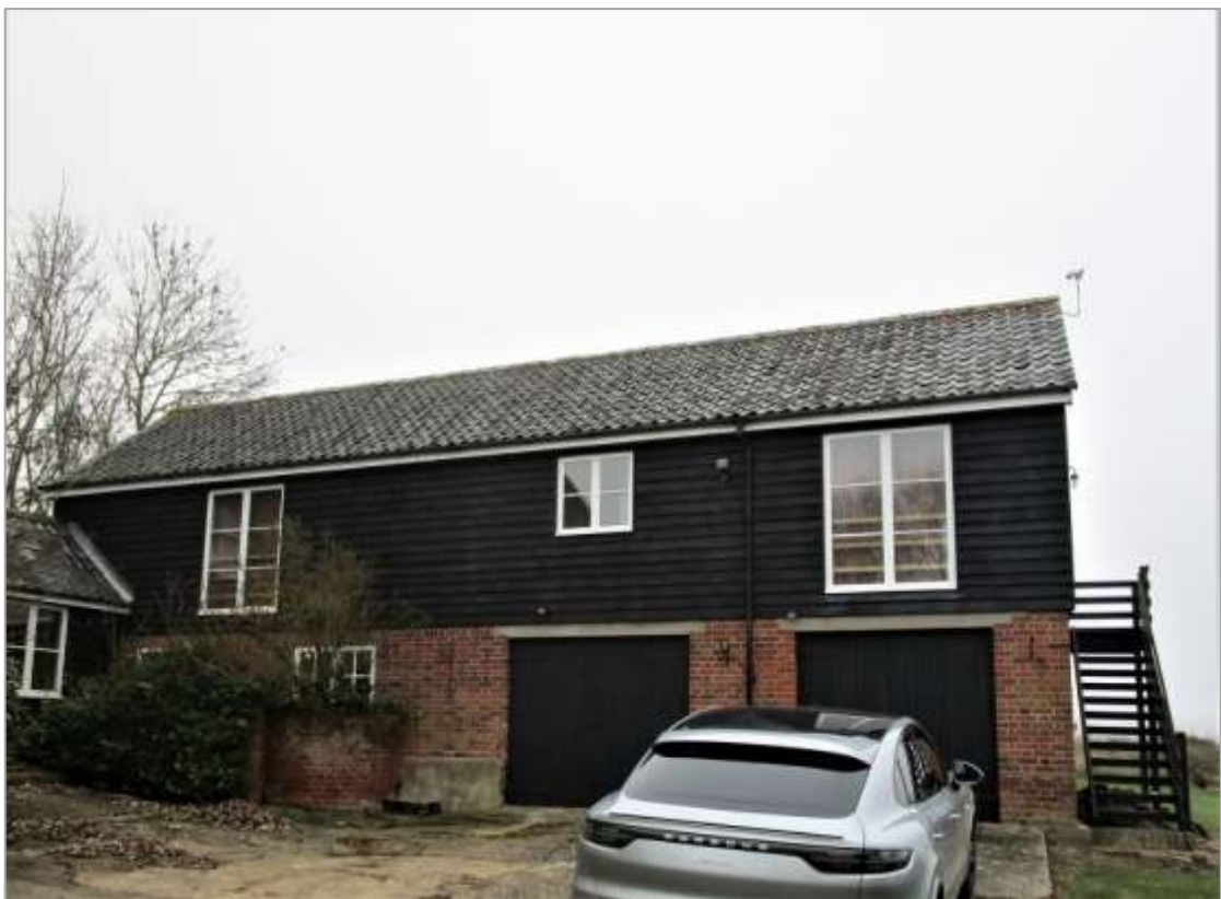
Fig. 20: S elevation of the N range (Building B), which originated as a single-storey cow house. A forebuilding, possibly timber framed, lay in front of this elevation. The main structure was built of brick, and some original brickwork survives. Most was renewed in Flettons in the C20, and in c.1990 the building was much altered, with a timber framed and weatherboarded upper storey and new windows and garage doors.
