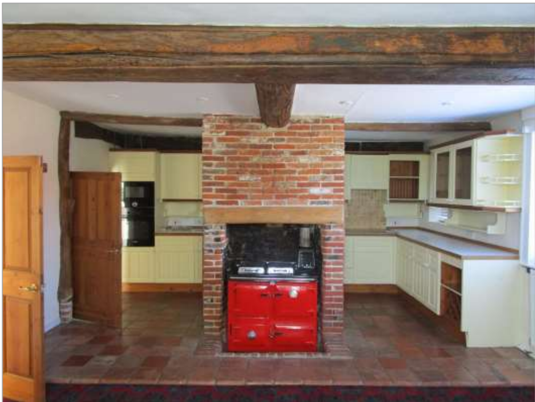
Fig. 17: Ground floor of 'cross wing' looking N, with moulded and chamfered spine beam and inserted C19 stack.
