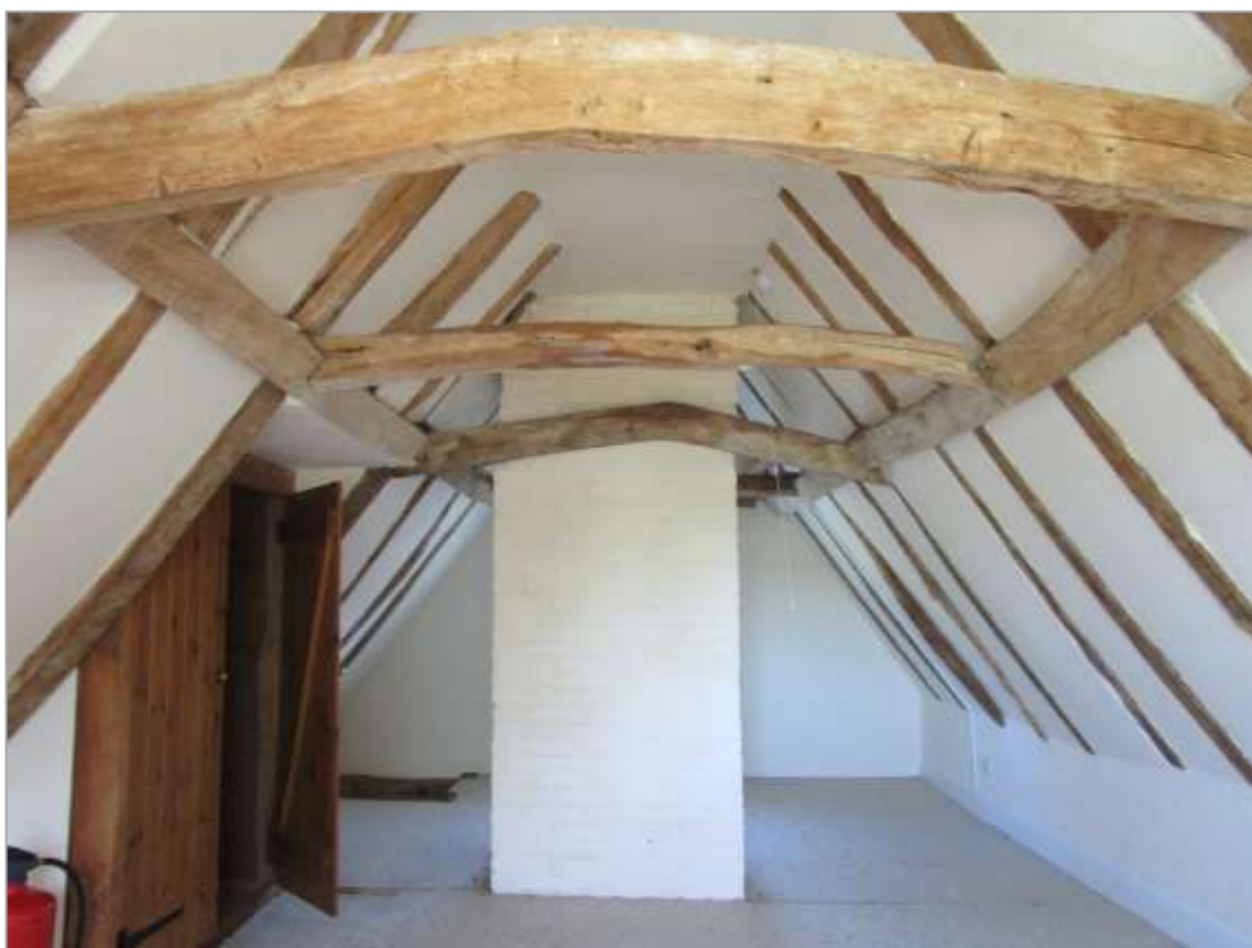
Fig. 19: Cross wing second floor, looking N, with collar purlin roof and inserted C19 stack
