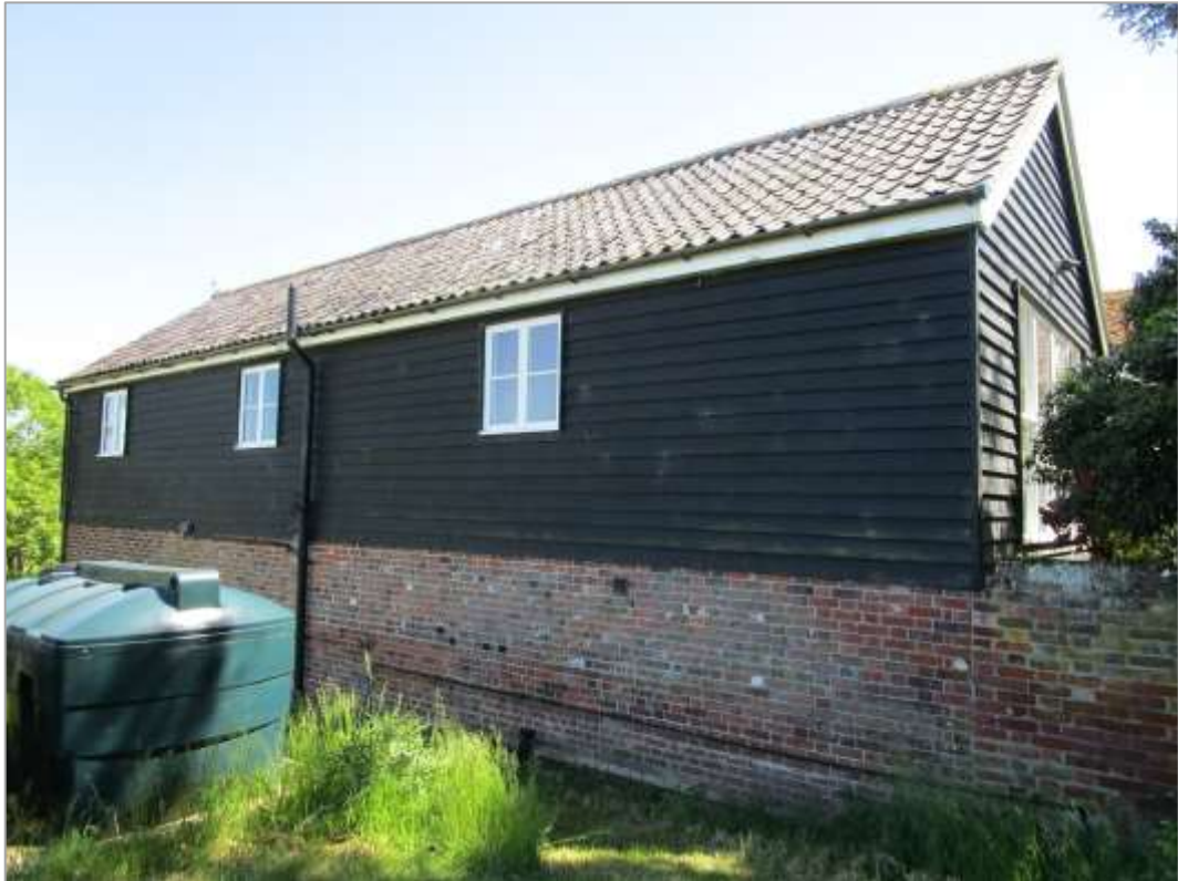
Fig. 21: The N elevation of the N range, showing C20 brickwork on the ground floor. The upper floor dates from c.1990.
