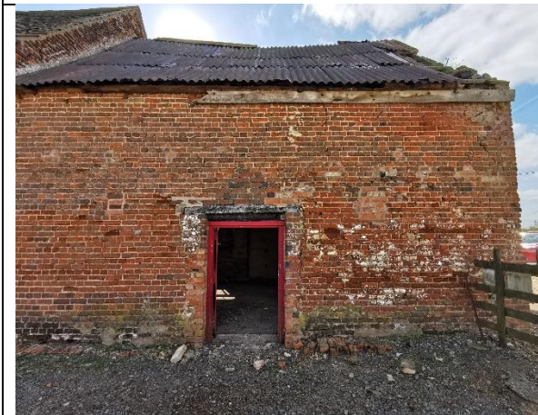
TN5 Gaps behind wooden fascia panel SW S1.
