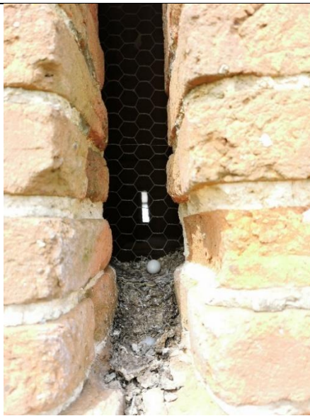
TN9 Ventilation slits leading directly into S1 (also used by nesting doves).
