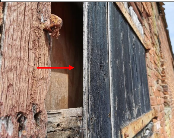
TN17 Gap behind wooden panels of door / eastern end of SE Face S1.
