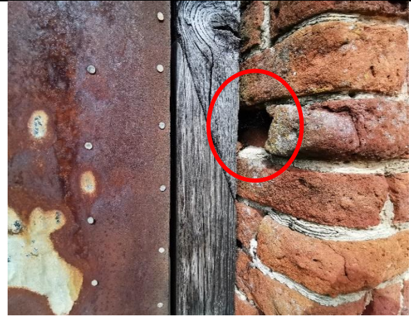
TN14 Gaps between door frame and brickwork SE S1.
