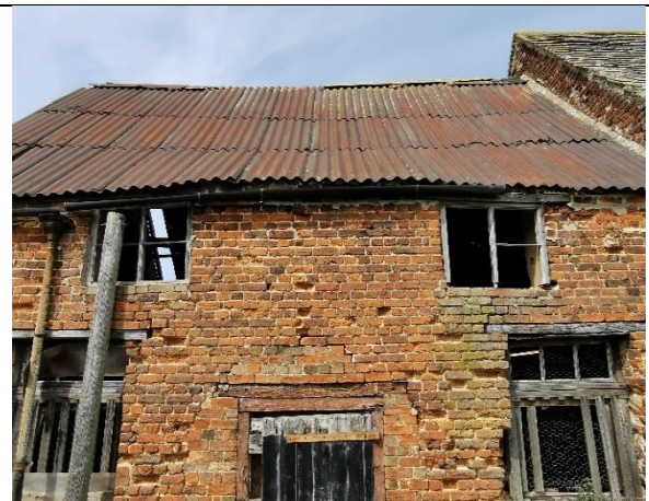
TN16 Missing panes in windows SE face of S1.
