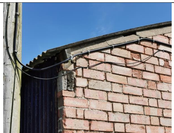
TN28 Degraded concrete under asbestos roof panel.
