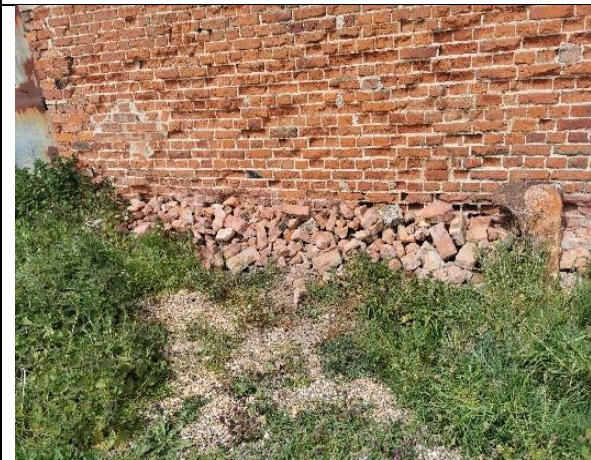
TN39 Fallen bricks.
