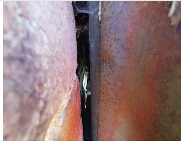
TN32 Gaps behind steel wall panels S2.
