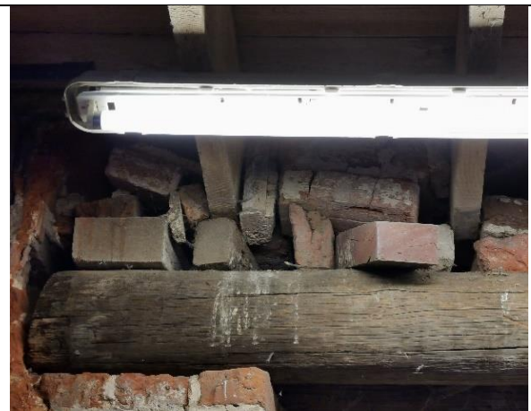
TN24 Loose bricks SW end internal S1.
