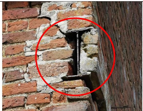
TN12 Gaps between steel girder and brickwork.
