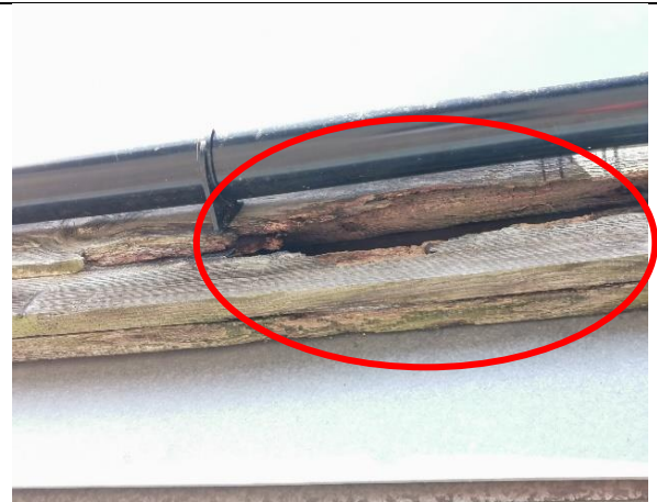
TN26 Rotten timber roof supports S2.
