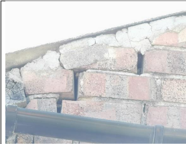
TN31 Gaps between brickwork S2.
