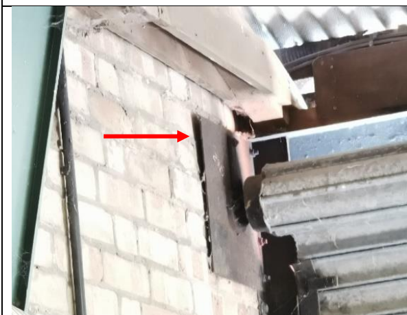
TN35 Gaps behind items stored against walls S2.
