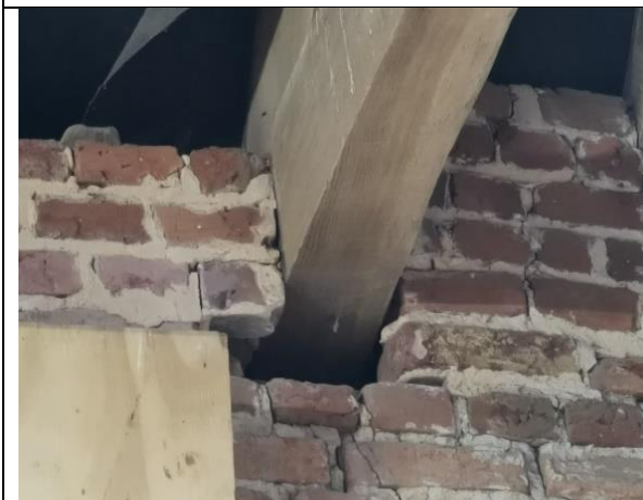
TN21 Gaps in brickwork around timber supports, internal S1.
