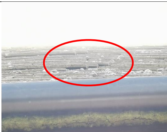
TN11 Gaps under lifted tiles S1.
