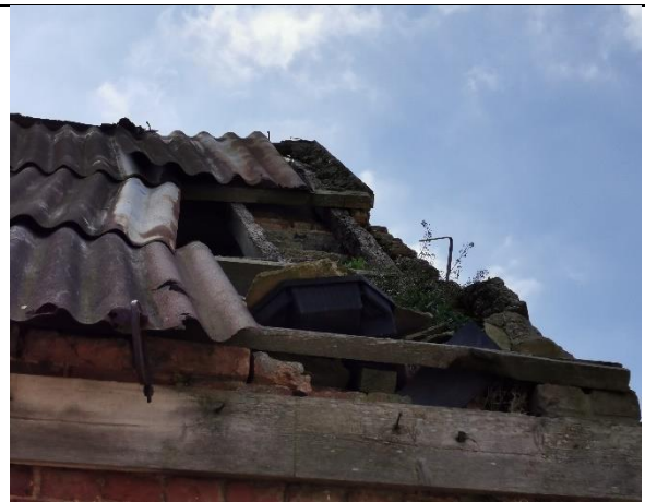
TN4 Missing roof panels SW end S1.
