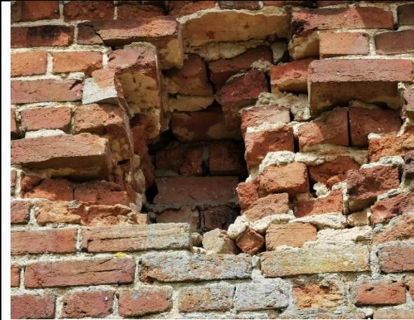
TN13 Large cavity of missing bricks, SE corner of S1.
