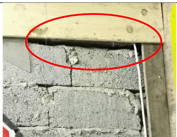
TN36 Slight gaps above breeze block wall S2.
