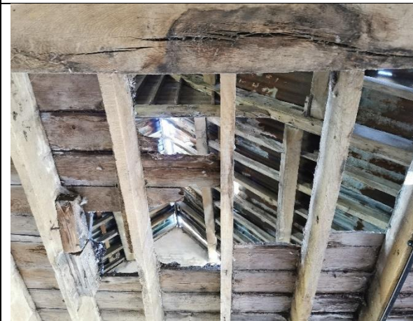
S1 – Unstable ground floor ceiling of SW end.
