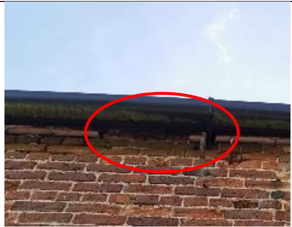
TN8 Felt degraded and missing between wood and brickwork NW aspect S1.
