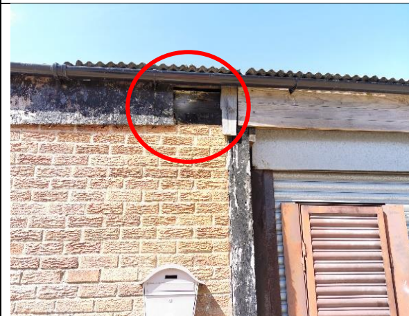
TN29 Rotten fascia boards S2.
