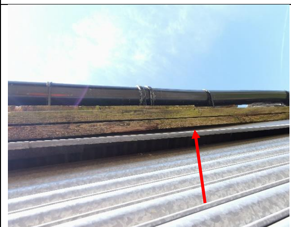
TN27 Gaps behind fascia board.
