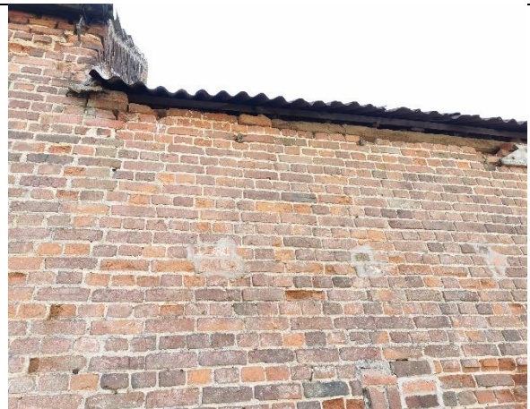
TN6 Missing bricks along top course western end S1.
