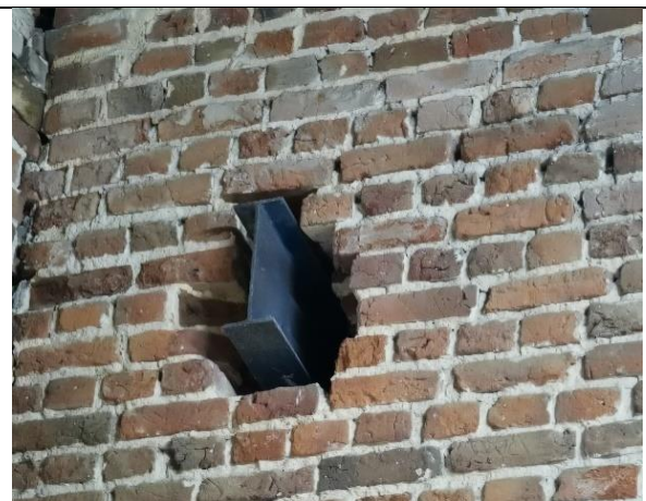
TN22 Gaps around steel girders internal S1.
