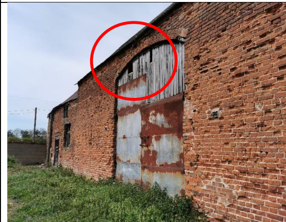
TN15 Gaps between wooden panels of door, providing access points, SE S1.
