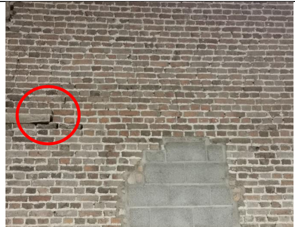
TN20 Gaps between wooden lintel and brickwork internal S1.
