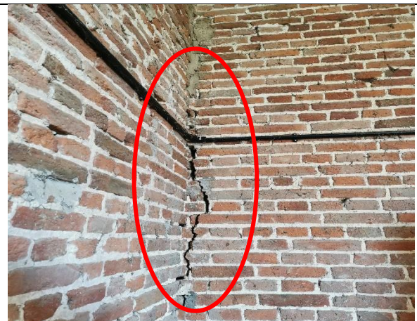
TN18 Multiple cracks in internal brickwork S1.
