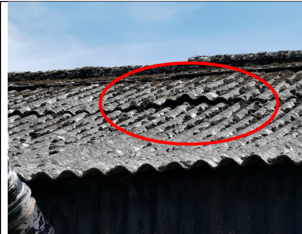
TN25 Gaps under roof sheets S2.
