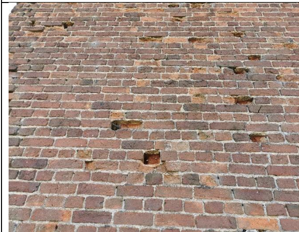
TN3 Degraded brickwork across whole of S1.
