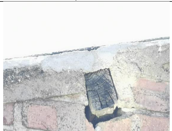
TN30 Gaps between timber support & external brickwork S2.
