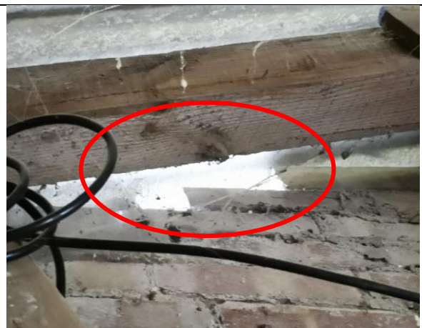
TN34 Missing bricks S2.
