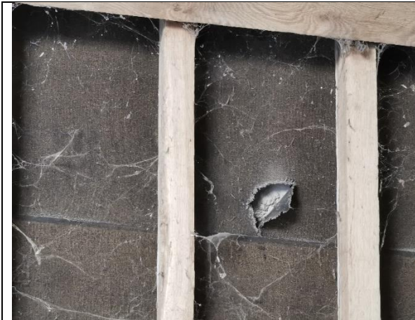
TN19 Tear in felt lining eastern end internal S1.
