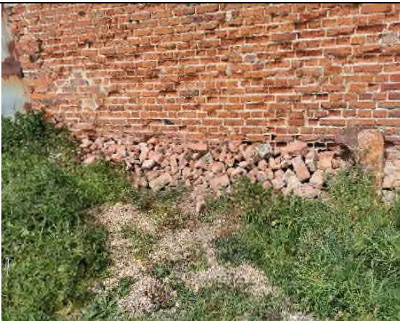
Loose bricks – TN3.
