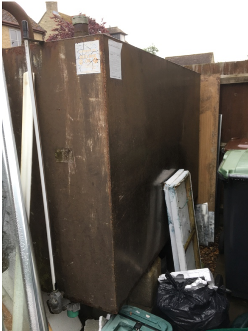
Existing oil Tank
