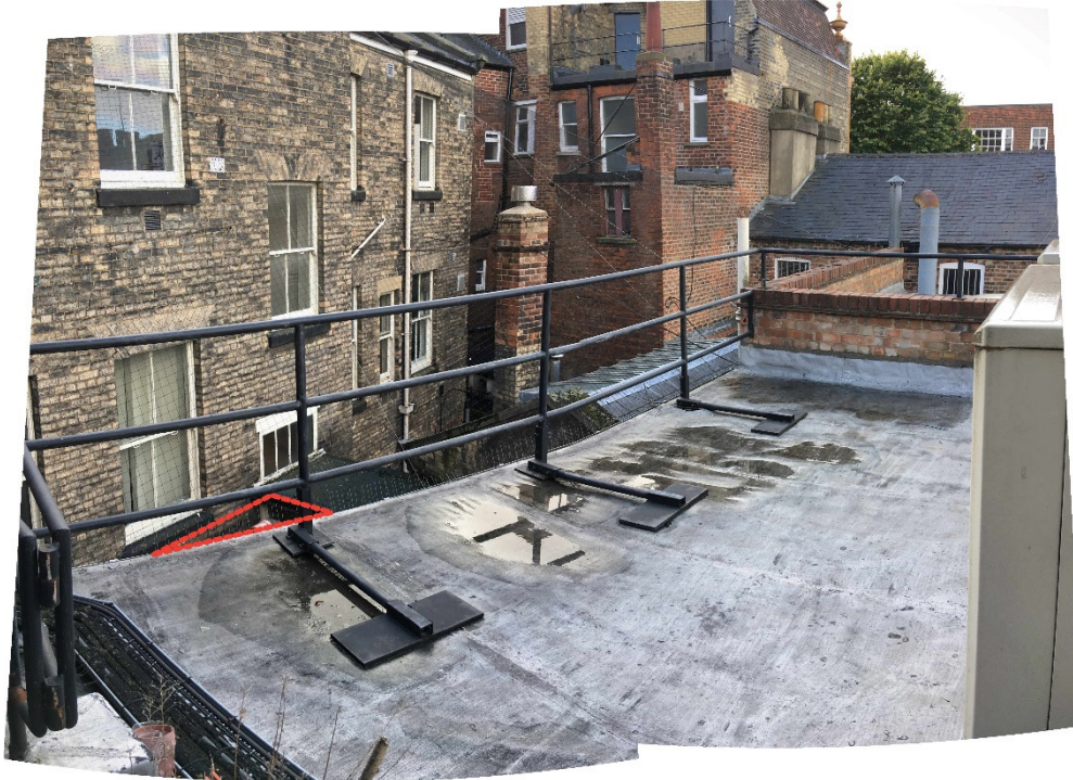
View of the Courtyard from roof of adjacent building (to North East of courtyard). Top of proposed plant denoted in red
