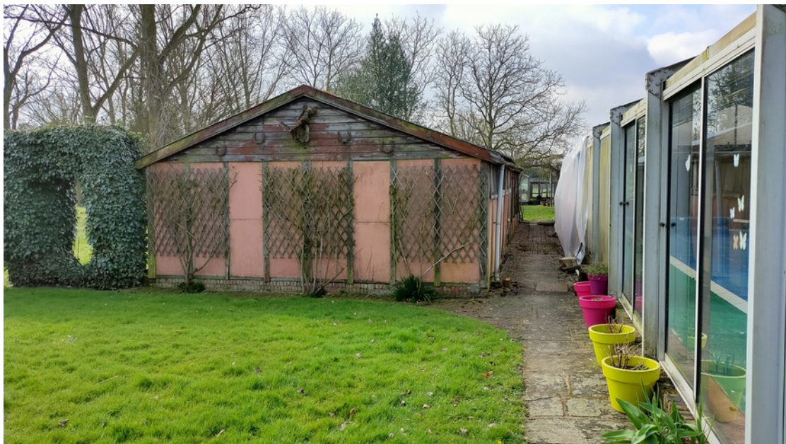
Unused outbuilding to be converted to changing rooms. Pool building to RH
