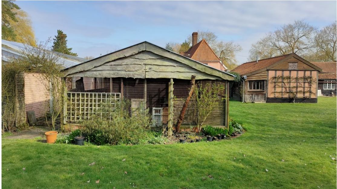
South end of outbuilding to be clad, glazed and used as potting shed and for pool pump equipment
