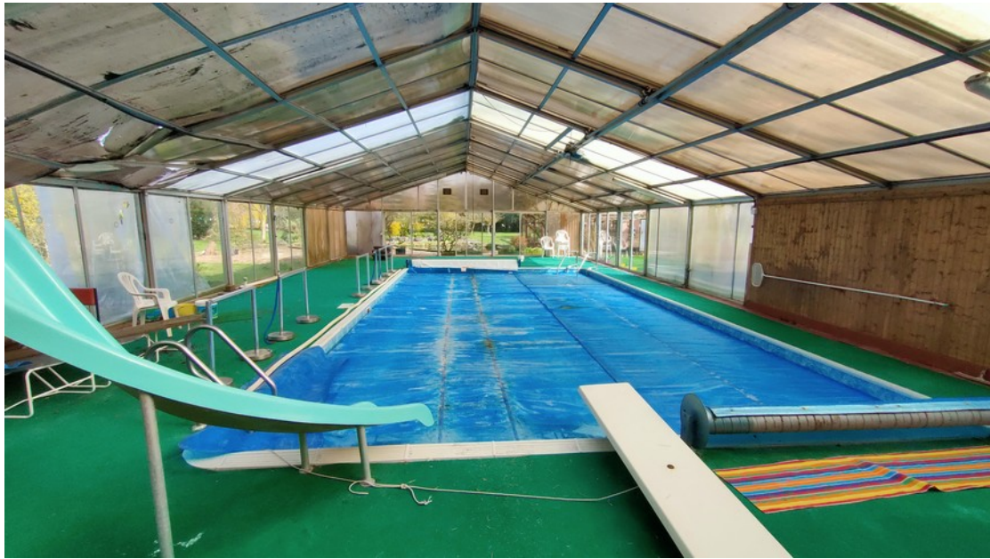
Internal view of pool building. Damaged frame clear.
