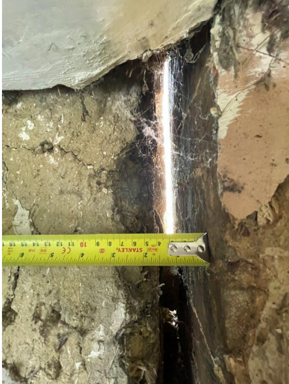
Crack between masonry chimney and clay lump
