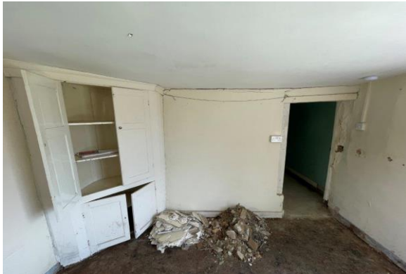
Interior ground floor facing east, cupboard to corner, formed off damp floor timber deteriorated
