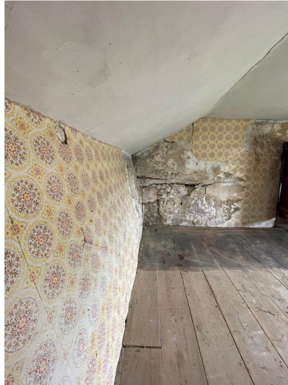
Photo of north wall showing extent of lean/splaying of roof structure to first floor walls
