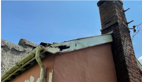
Timber has deteriorated throughout
