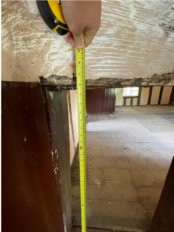
Low level doorway, height determined by existing wall plate to main house.
