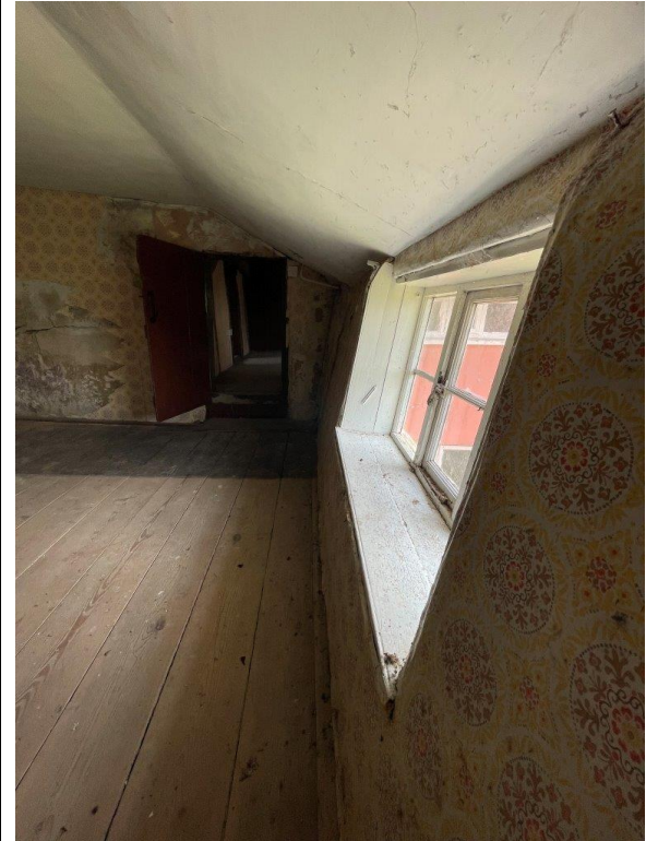
Photo of south wall showing extent of lean/splaying of roof structure to first floor walls
