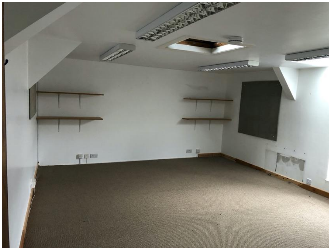
Figure 16: Area of false ceiling in Unit 7 (first floor) to be removed to expose rafters
