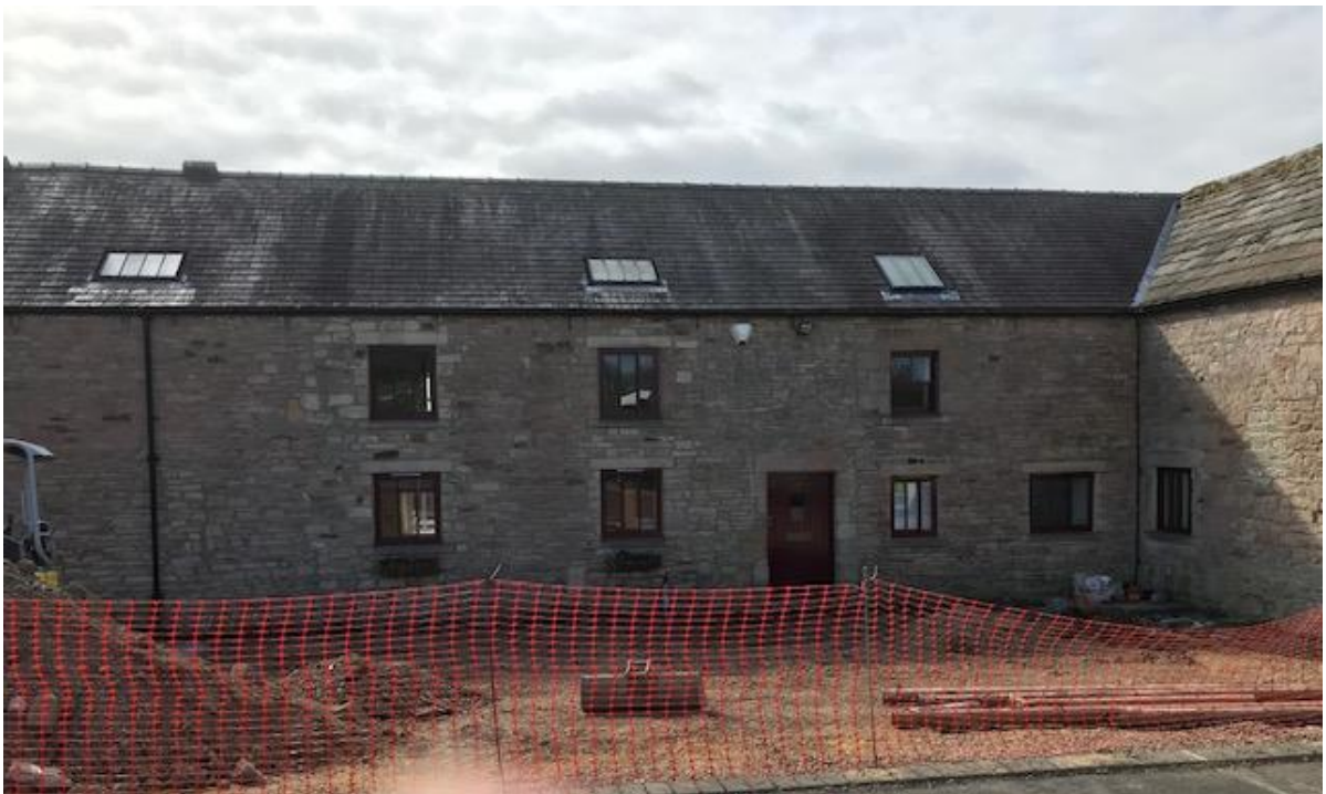
Figure 4: Parking areas to the front of Unit 7 (currently works in place for drainage purposes)
