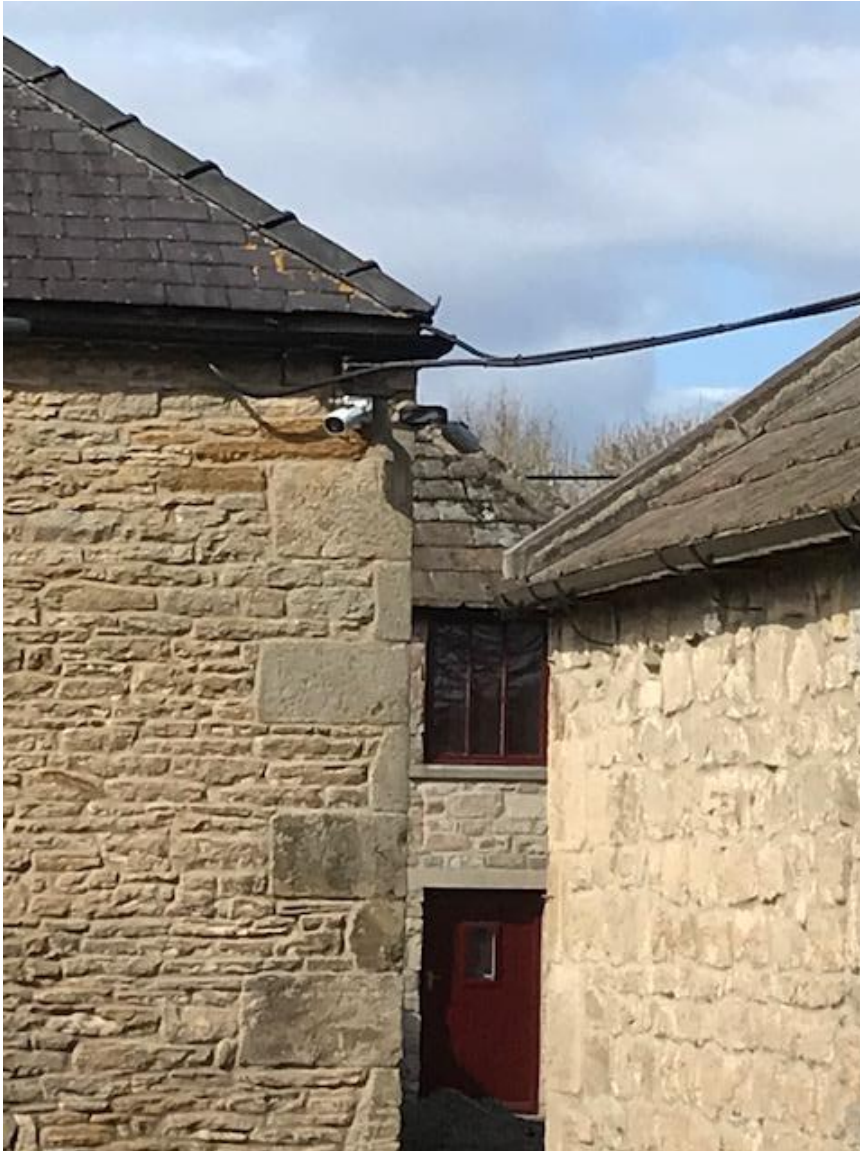
Figure 10: Camera 3: CCTV Unit to front of Unit 7
