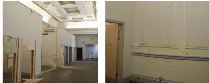
A Modern stud partitions have altered the proportions of the space and damaged the historic fabric
