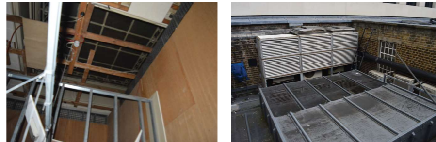
B The false roof and service void hides the skylight, which is concealed by a lead finish
