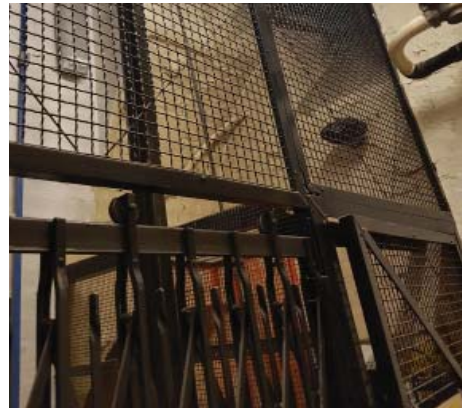
Photograph showing service lift caging
