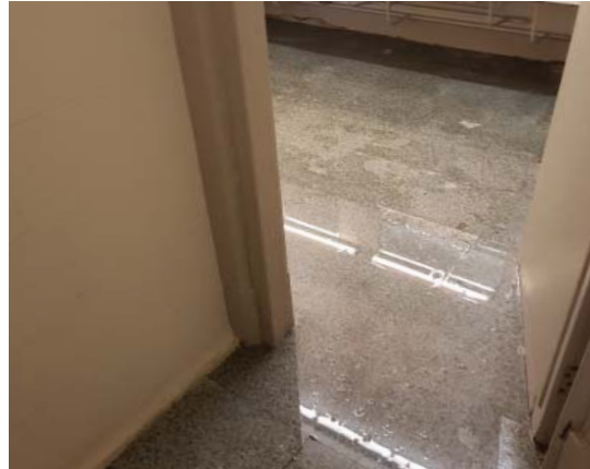
Photograph showing flooding to toilet areas
