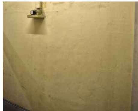
Photograph showing cracked outline of historic door
