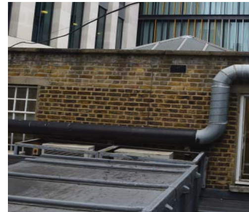
Photograph showing change in brickwork suggesting the roof level and parapet walls have been altered
