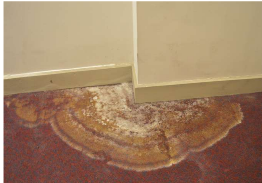
B: Excessive mould beginning to grow around floor slab
