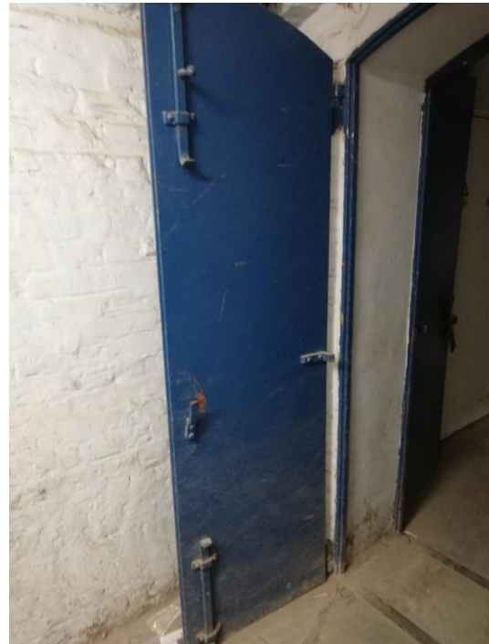
Image 26 (above) and Image 27 (right): Original cast iron doors for security and fireproofing within basement
