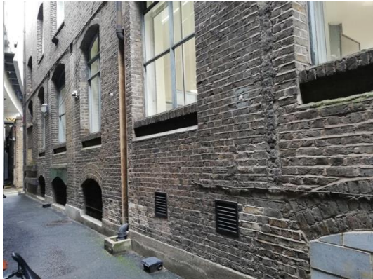
Image 79: Filled basement lights, and altered windows.
