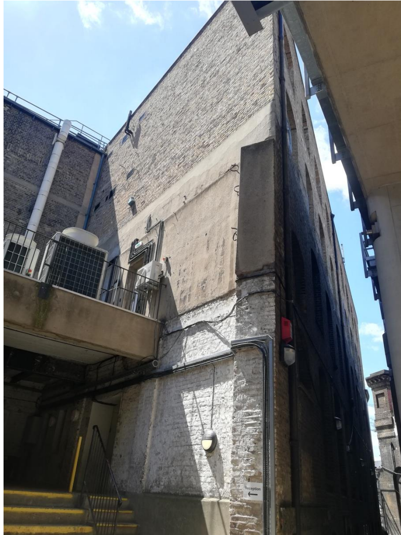
Image 78: Elevation 10 showing original parts of surviving walls at base with new brickwork over
