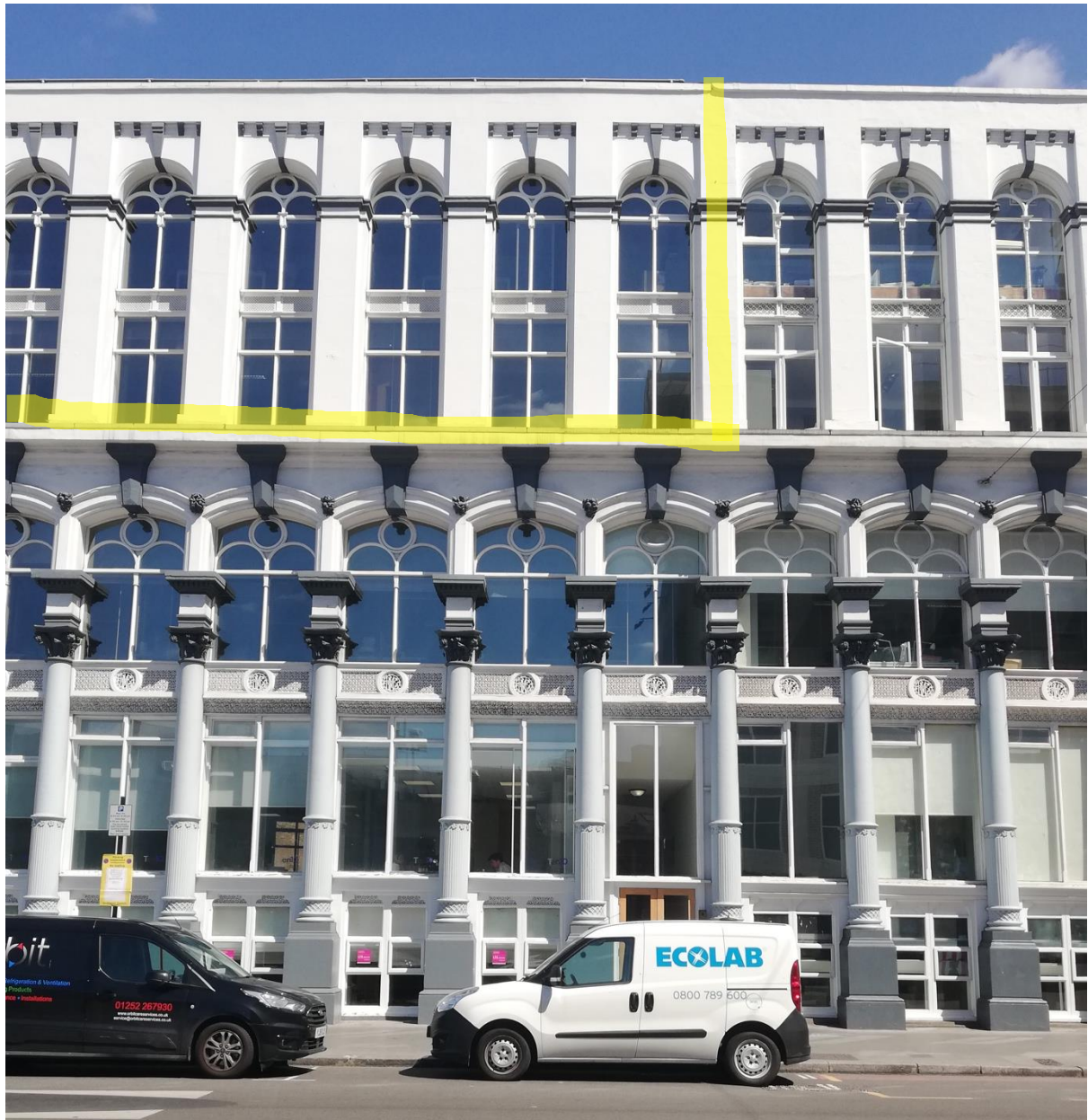
Image 65: West End with areas of new construction above and to the left of highlighted line
