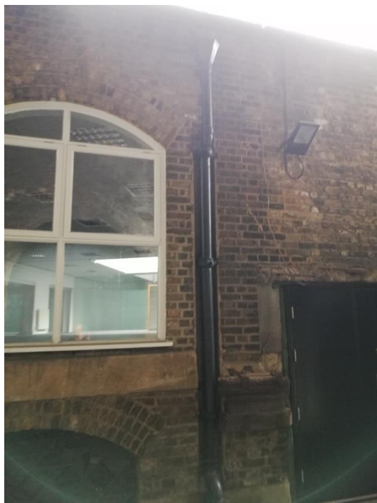
Image 75: Early lower part of wall with Atrium Suite over. Door to lower ground floor archive.
