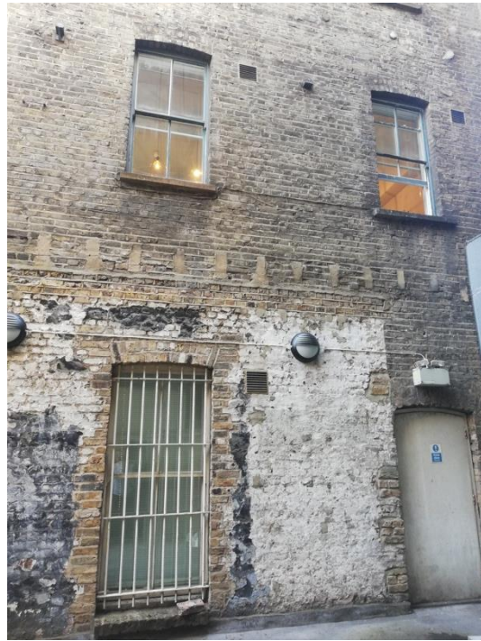
Image 73: This image of the lower part of this wall shows possible fire damage to brickwork, the location of infilled joist holes and the creation of a new opening.
