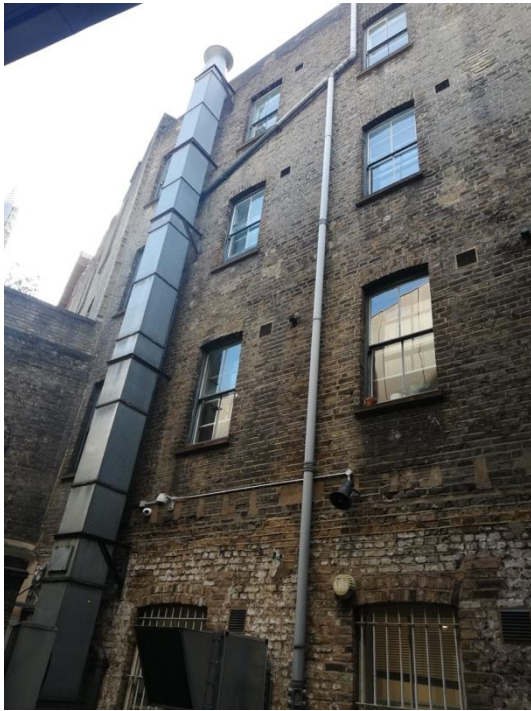
Image 72: Originally internal walls, these were exposed after demolition of the rear hop warehouse after the 1920 fire, and windows inserted into the original atrium offices.
