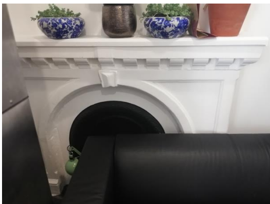
Image 39: Original Fire place – ground floor, this is typical of many that survive throughout the building
