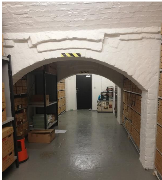
Image 28: Archive with original soft floor forms cellar area beneath north south run off trading floor offices
