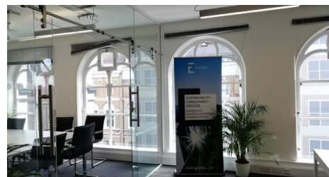
Image 55: The use of glass and lightweight ducting allows the form and shape of the original windows to still be appreciated
