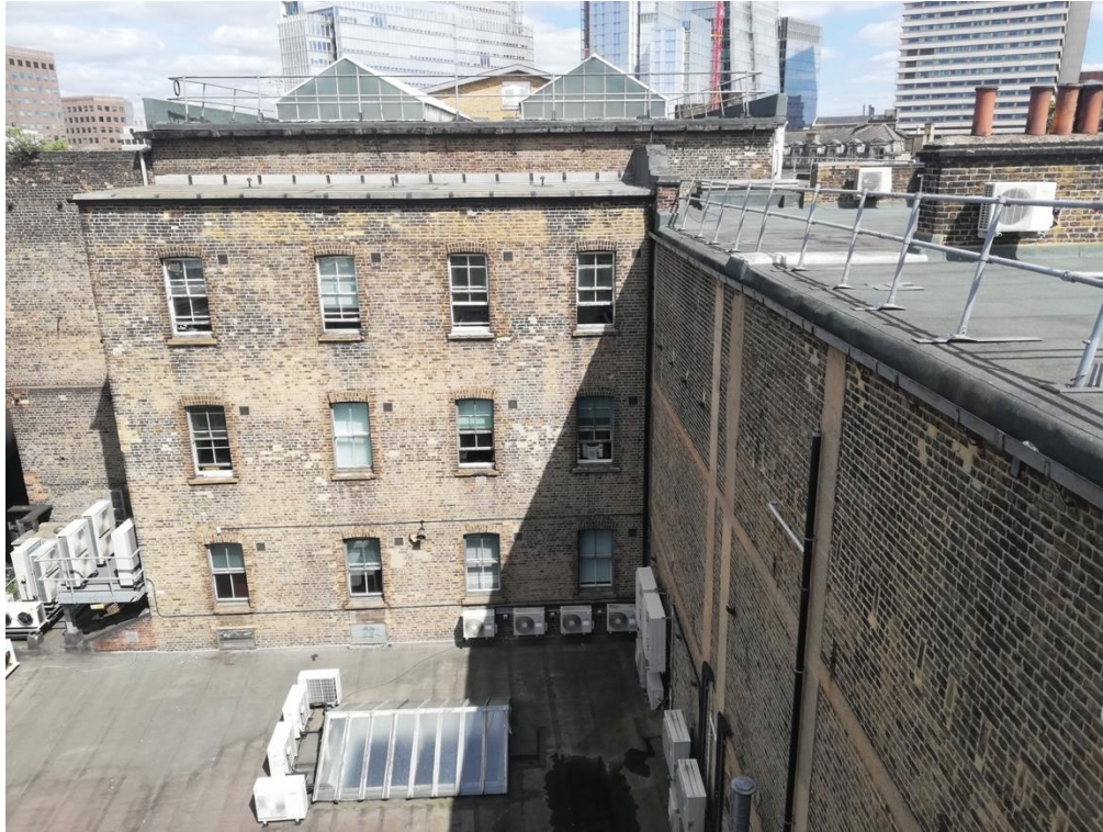
Image 74: Elevation 8 with sash windows inserted into Trading Floor offices after the 1920s fire
