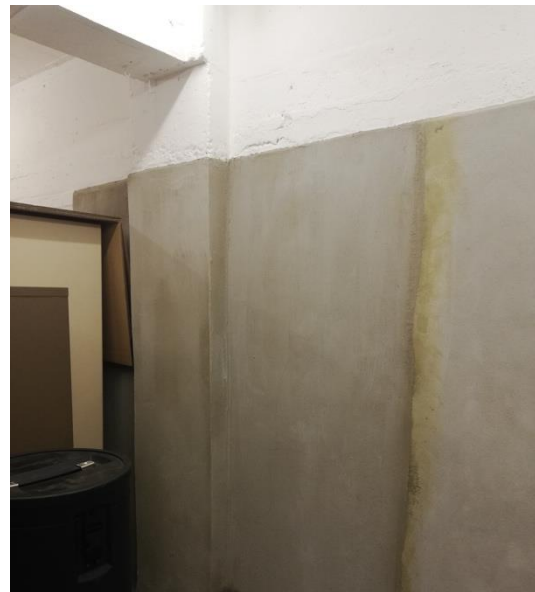
Image 29: Modern area of construction and tanking to north west side of archive and beneath atrium suite
