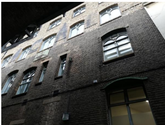
Image 81: Modern windows with new build clearly visible on top two floors with remodelled windows.
