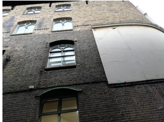
Image 80: Repair / new bricks forming vertical line below stucco
