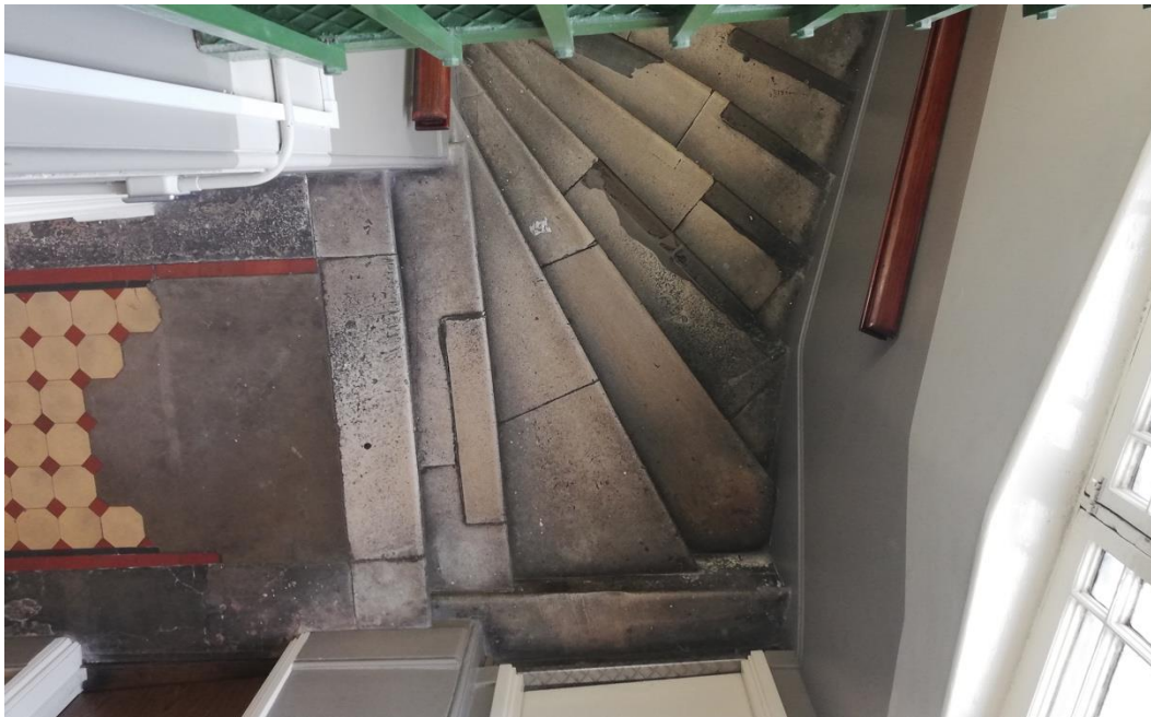
Image 58: View looking down NE stairwell which shows patina and texture formed by wear and tear and careful repairs over 150 years.
