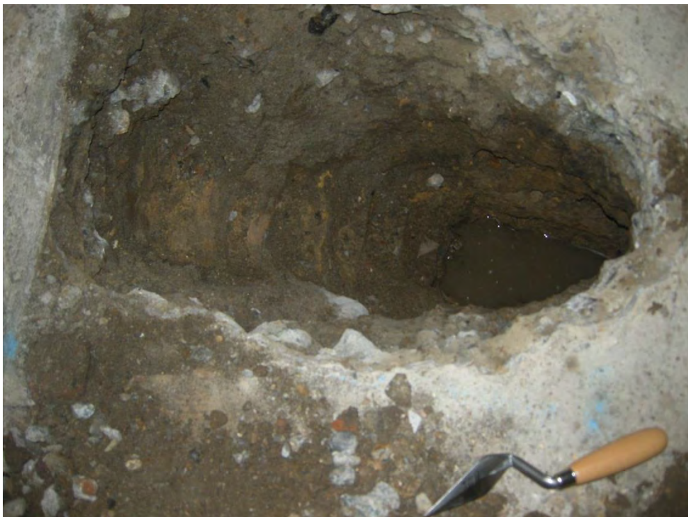
Photo 2 TP 2A, against a footing in a room in the lower basement, looking north-eastwards
