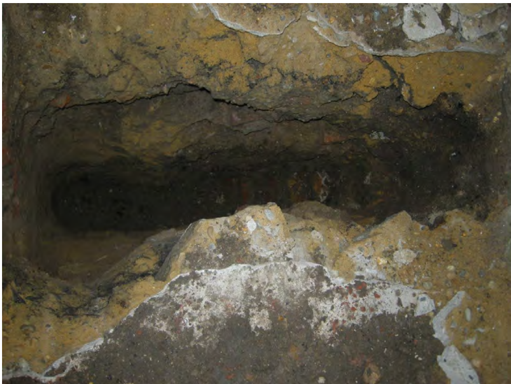
Photo 12 TP 11, in the coal cellar passageway, between the wall footings, looking eastwards
