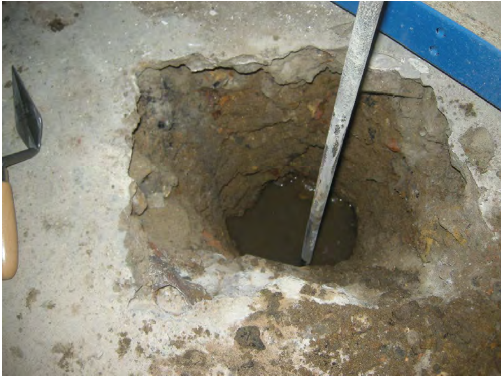
Photo 5 TP 4, against a central pier base in a room in the lower basement, looking south-eastwards
