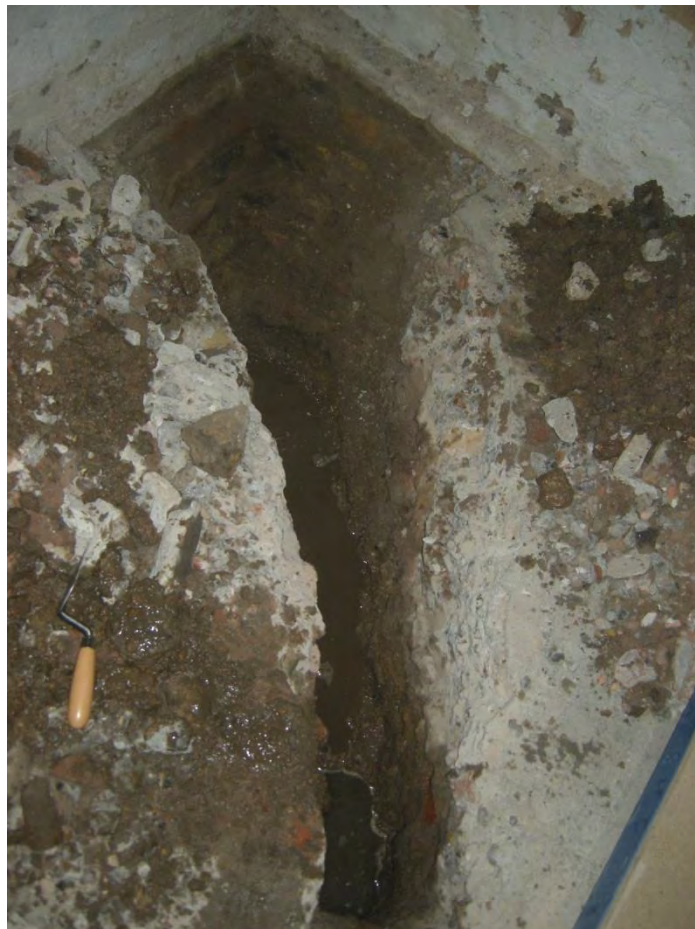
Photo 10 TP 9, against footings in the corner of a room in the lower basement, looking south-westwards
