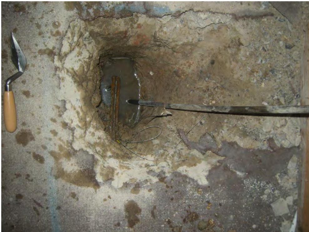
Photo 6 TP 5, against a footing in a room in the lower basement, looking eastwards
