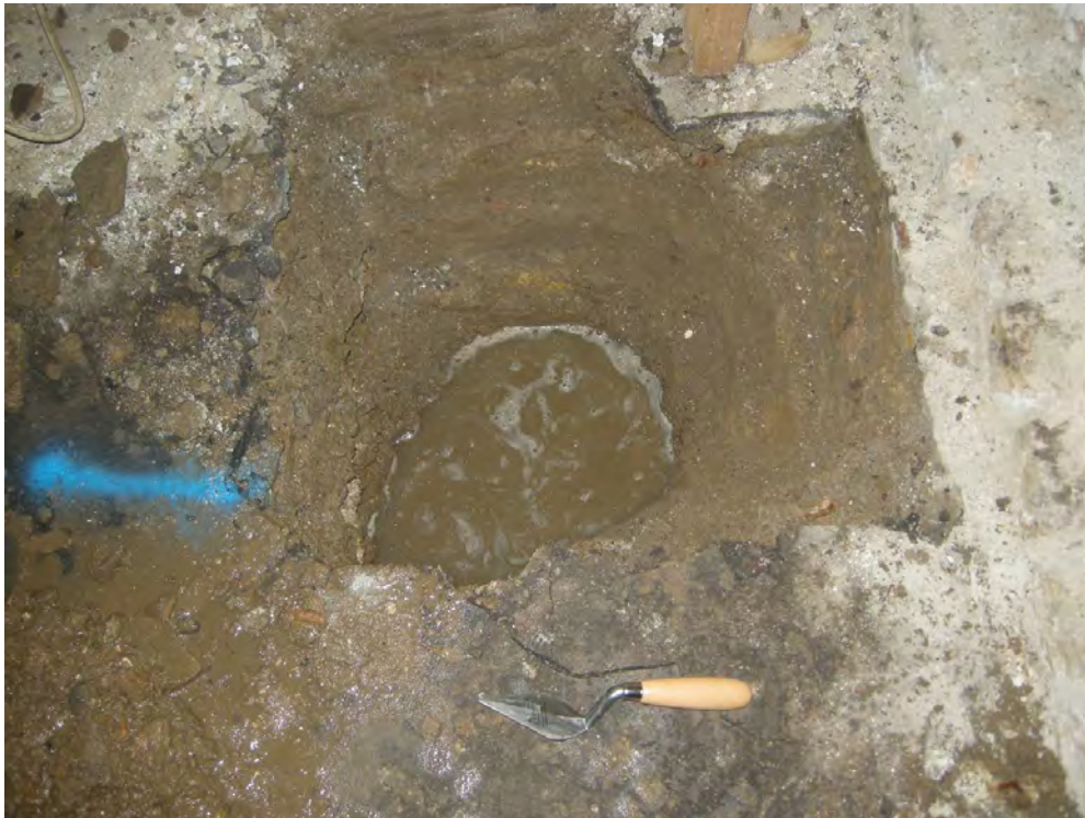
Photo 4 TP 3, against footings in the corner of a room in the lower basement, looking eastwards
