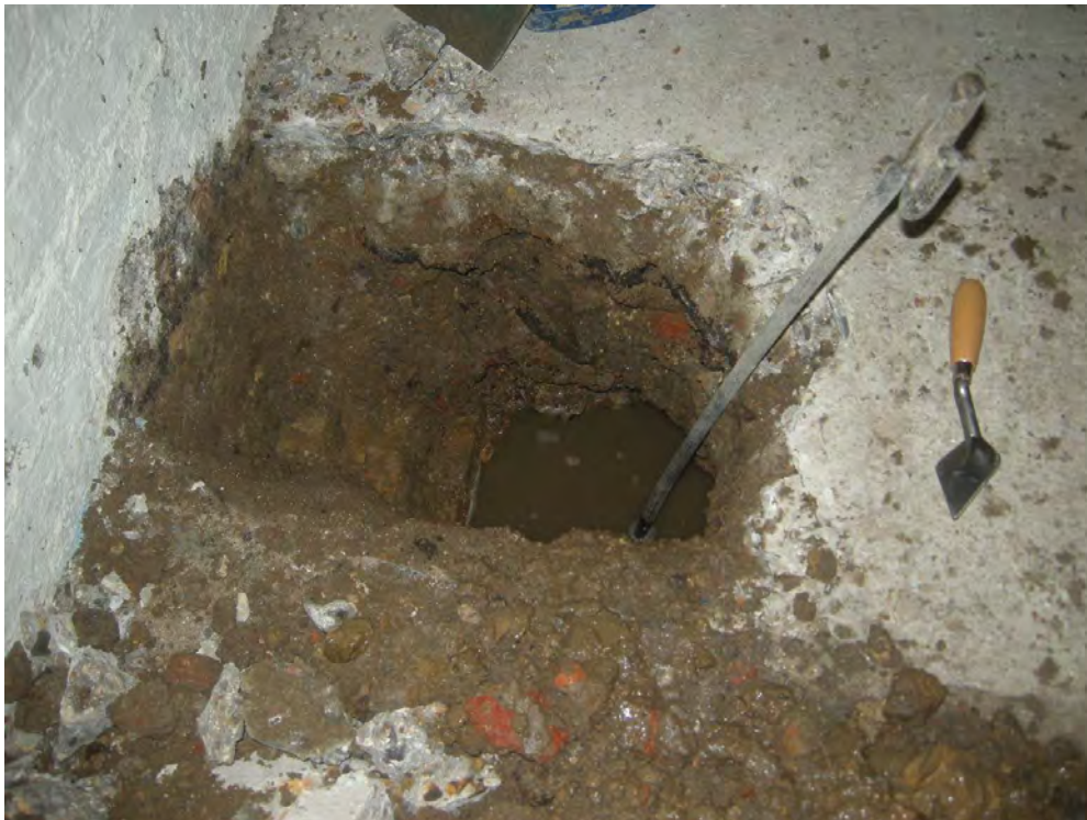
Photo 8 TP 7, against a footing in a room in the lower basement, looking eastwards
