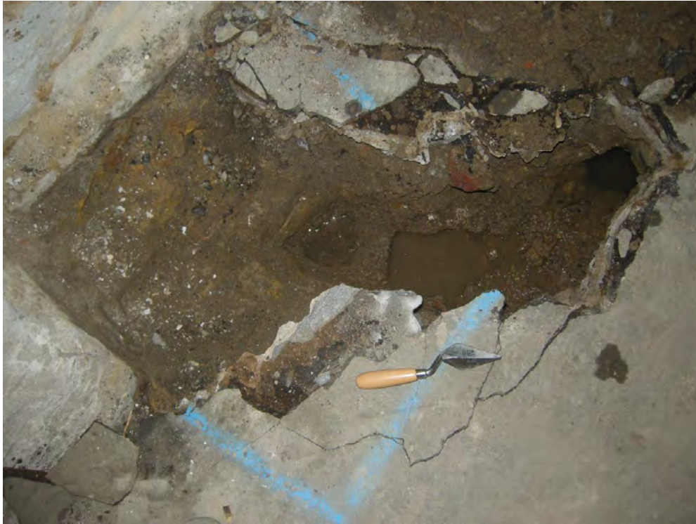
Photo 3 TP 2B, against footings in the central passageway in the lower basement, looking north-eastwards
