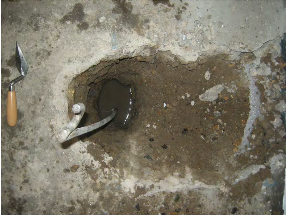
Photo 7 TP 6, against a footing in a room in the lower basement, looking southwards
