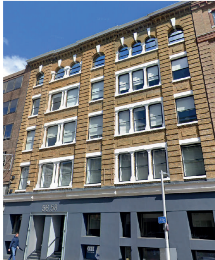
56-58 Southwark Street Yellow stock, parapet roof, arched windows, strong grid and rendered to the ground floor
