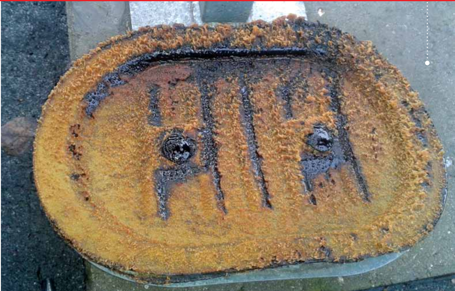
Inspection Hatch without JIMCO Technology - Not cleaned for 6 months
