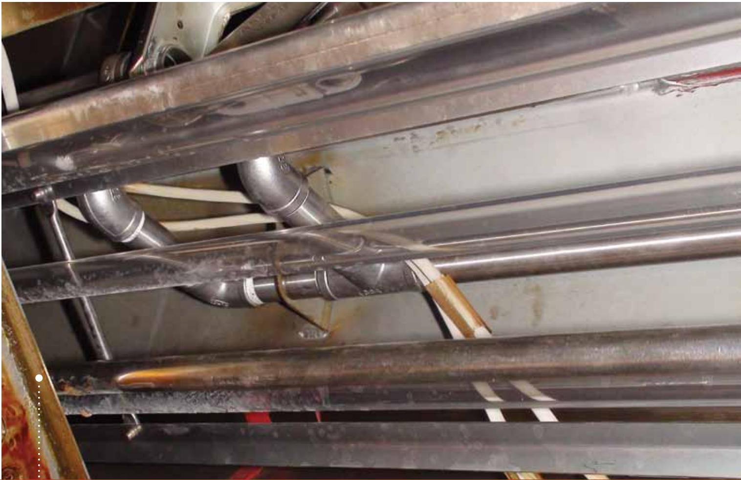
Hood with JIMCO Technology - Not cleaned for 6 months
