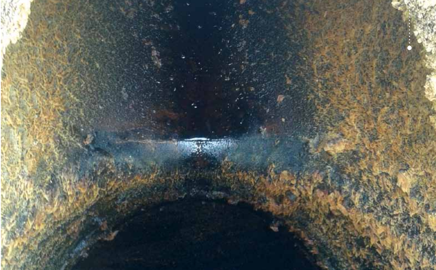
Duct without JIMCO Technology - Not cleaned for 12 months
