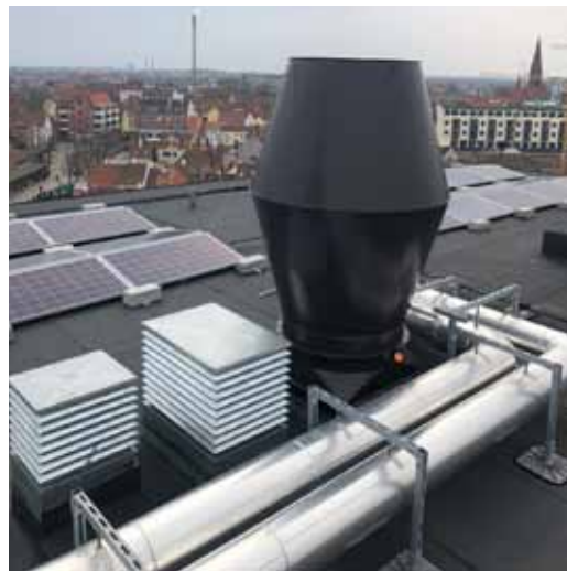
Air outlet from the kitchen
