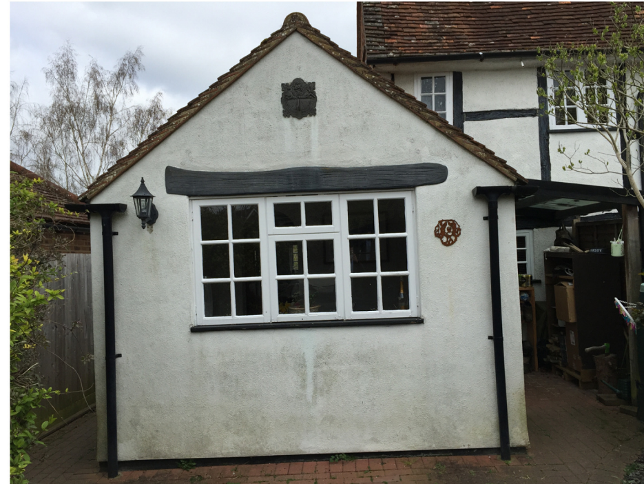
Existing timber window within 1990's extension. The window consists of white painted timber frames with a black painted timber sill.
