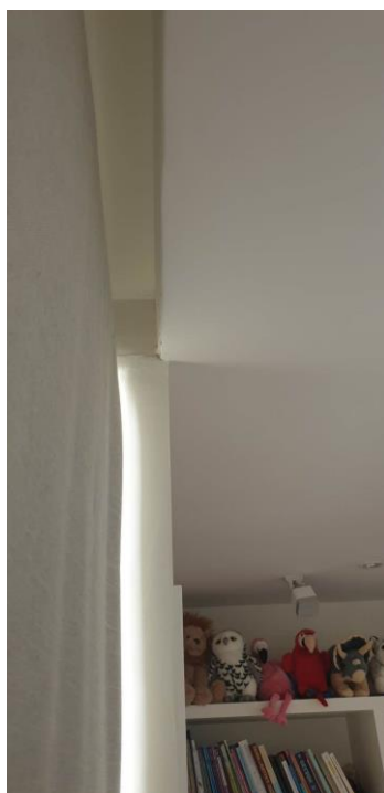
Evidence of Lowered Ceiling in Snug Room
