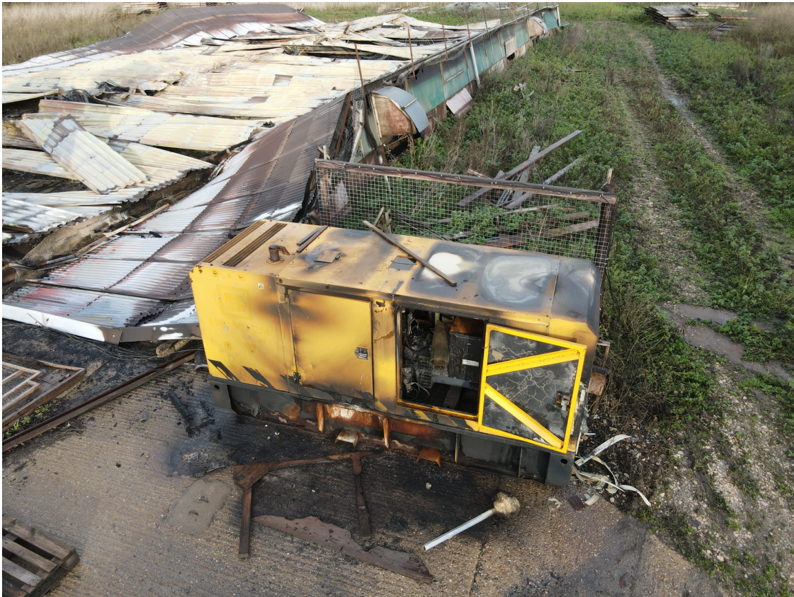
Picture 3 - Building after fire damage
