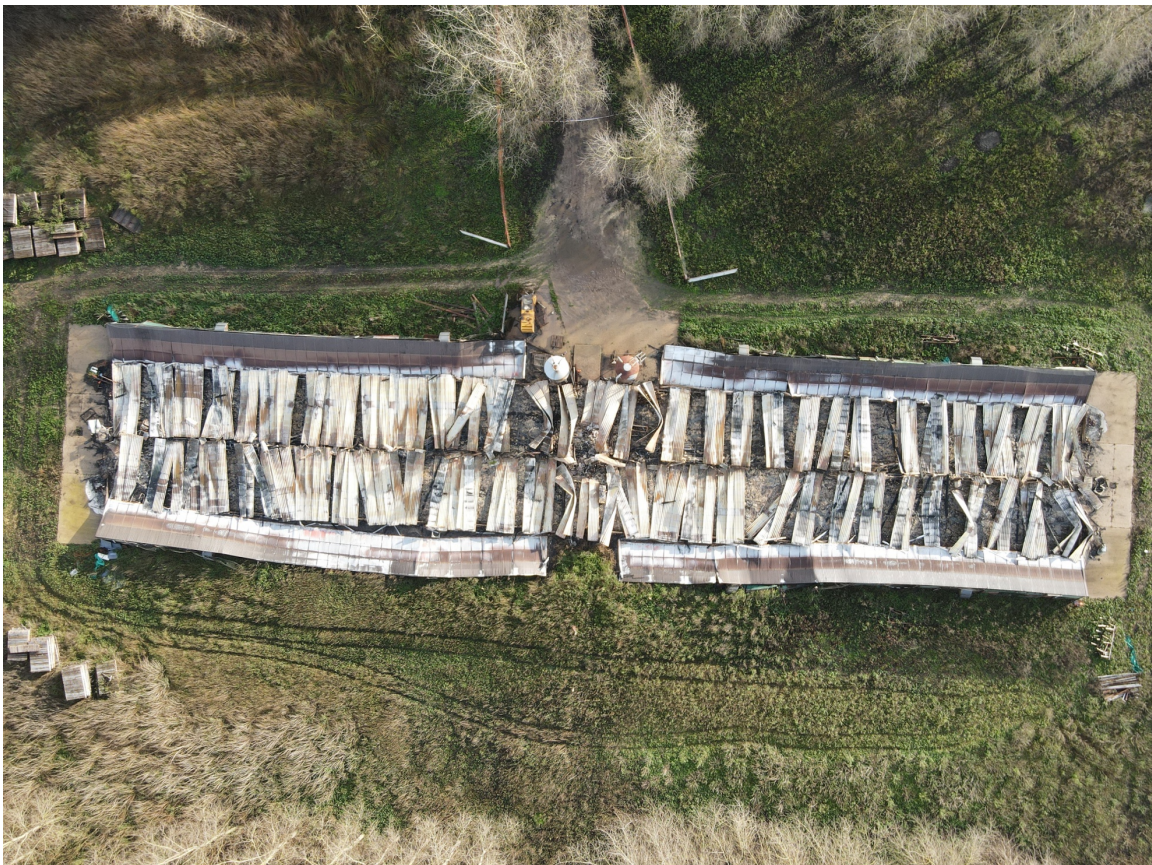
Picture 2 - Building after fire damage
