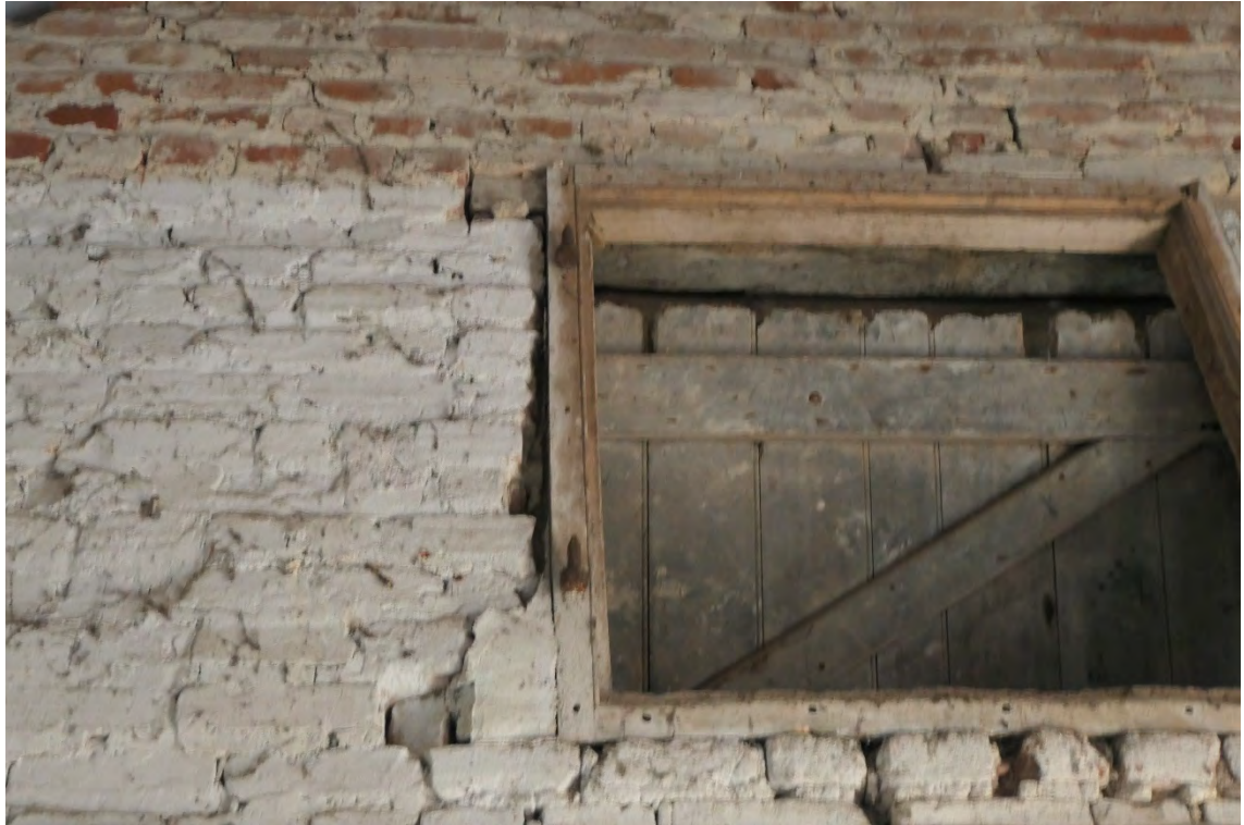
Photo 9 , gaps between brick and timber and within brick walls create ideal potential roost features.
