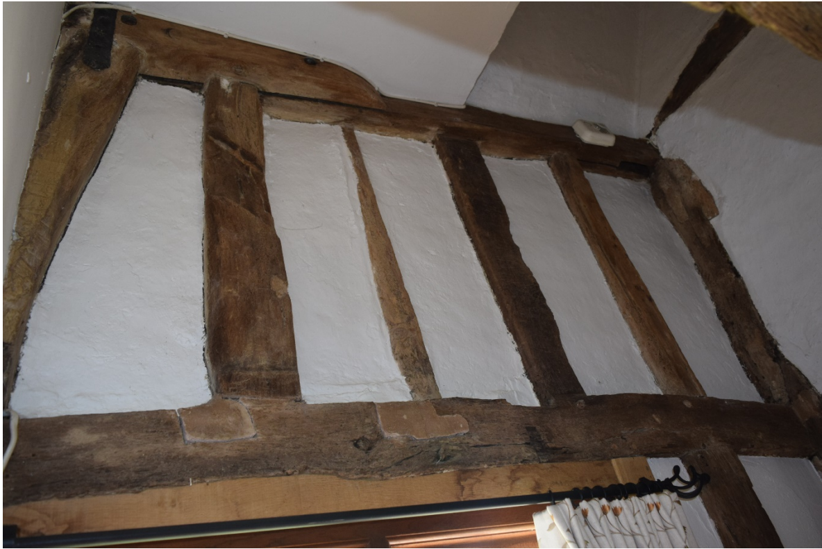
Figure 19: Reused timbers within the wall framing of the front wall of the cottage.
