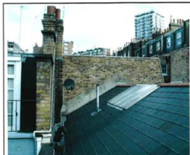
Figure 5 - View of existing roof looking north to party wall with 7 Connaught Close
