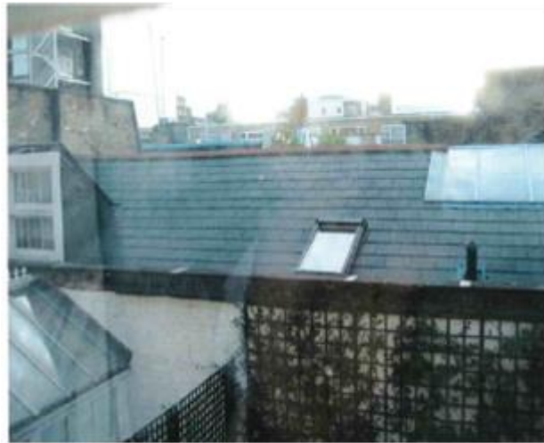
Figure 12 - View from 10 Albion Street looking west at the existing roof of the application site
