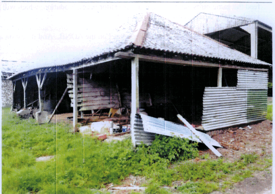
The Wagon Lodge with the 'Atcost' barn behind. Note the crude concrete stools supporting two of the oak posts and the remnant of the original weatherboarded end wall. There are no braces to the oak posts on the closest bay, so it can confidently be assumed that this part of the Wagon Lodge is an extension.
