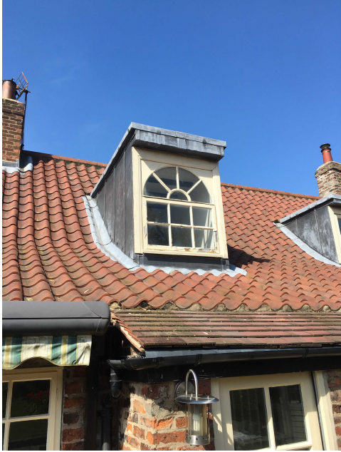
Photograph of the existing dormer window which, is in poor condition and is to be replaced.
