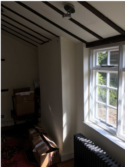
Photograph of the sitting room interior showing the existing disused chimney breast.
