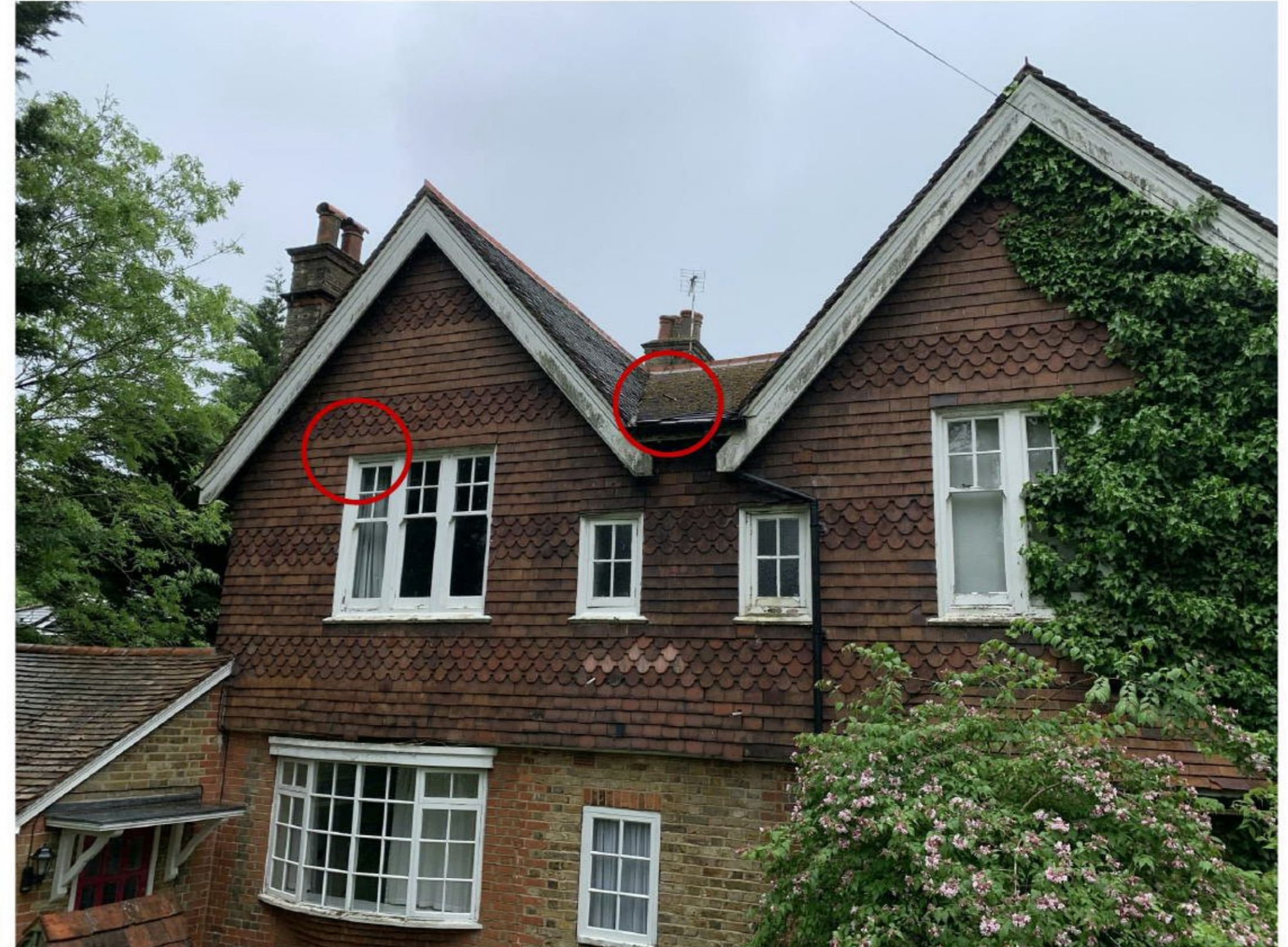
Photograph 2 – Northern aspect of B1. Cracked, slipped, and lifted tiles on front wall and roof.
