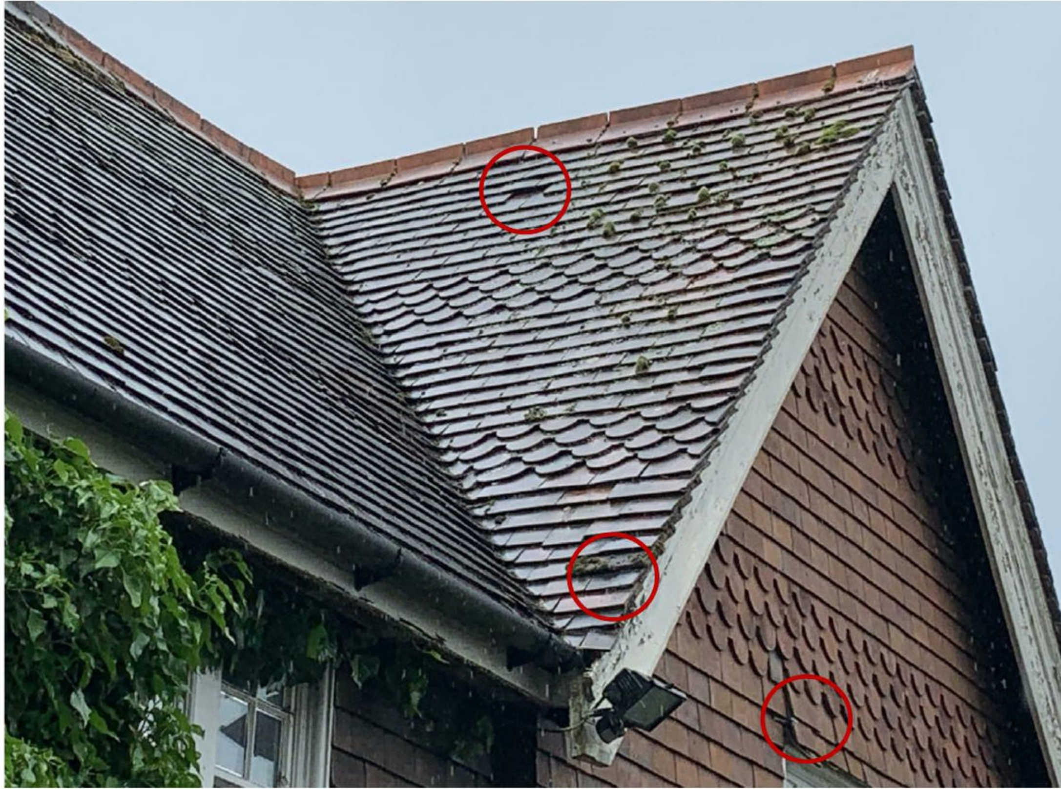
Photograph 1 – Western aspect of B1. Slipped tiles on gable roof, as well as lifted tiles above bedroom window
