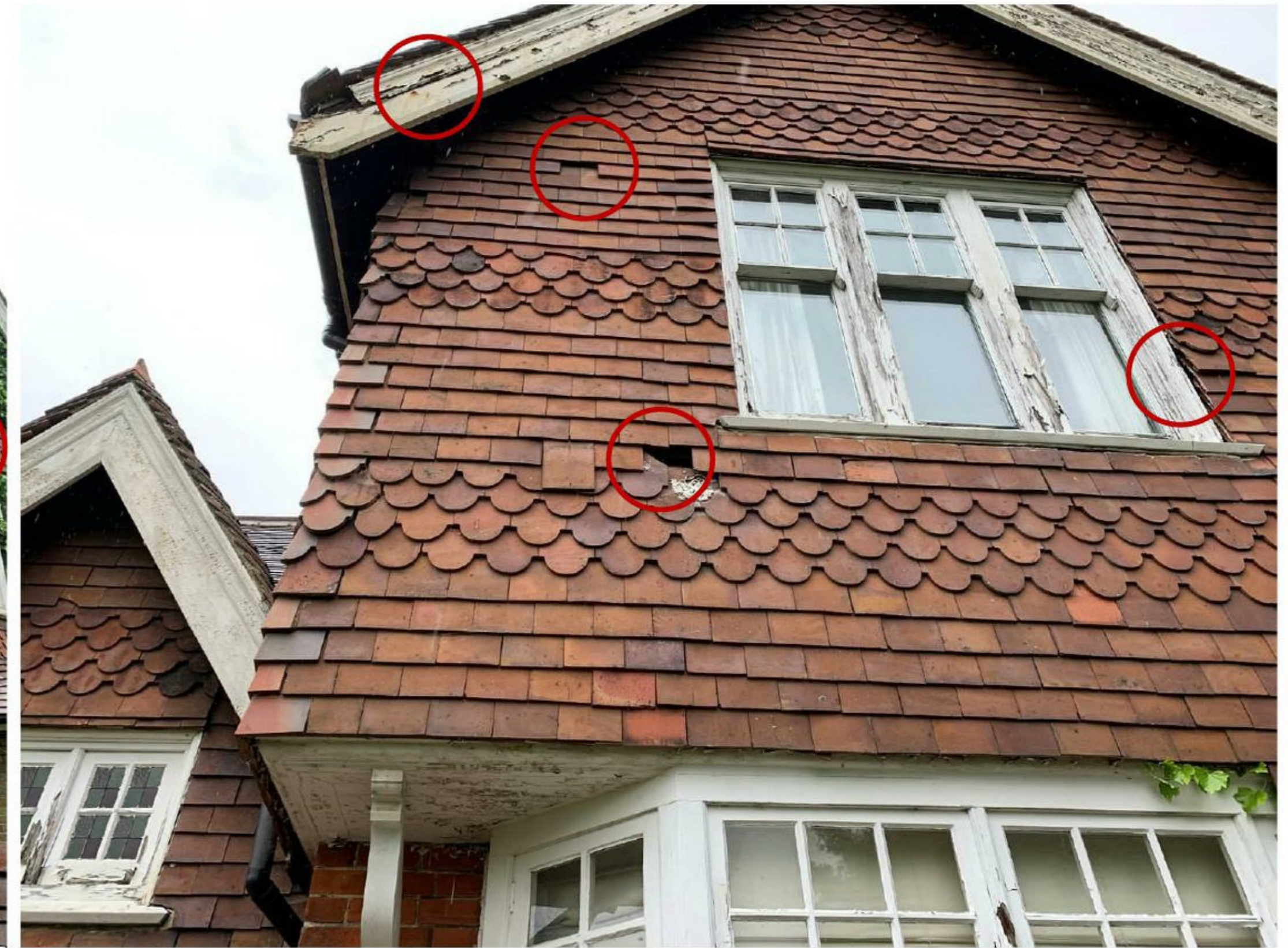
Photograph 4 – Southern aspect of B1 missing tiles evident beneath and adjacent to main rear bedroom window. Fascia board also in poor condition.
