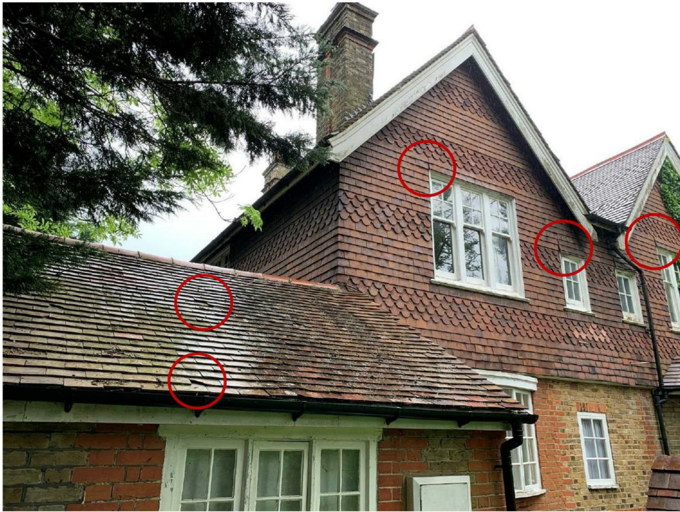
Photograph 3 – Eastern aspect of B1. Lifted tiles highlighted in proximity to bedroom windows. Note also slipped and cracked tiles over living room window
