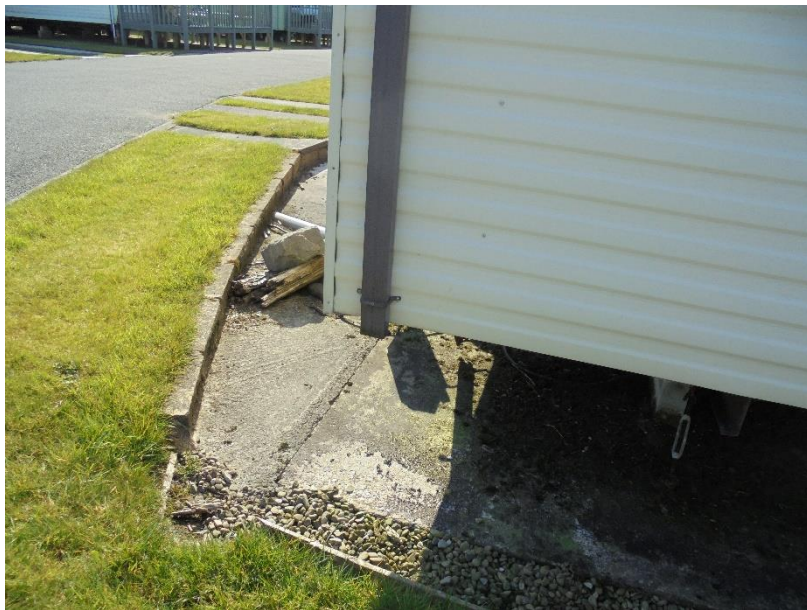
Photo 4: Example of existing surface water drainage with downspout to filter drain. However, not all the existing holiday homes have this arrangement.
