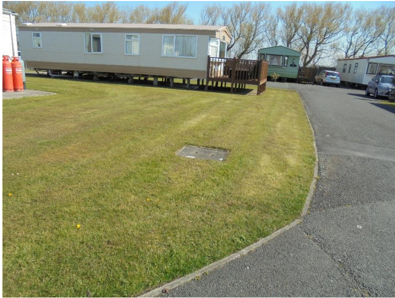
Photo 3: Existing foul drainage. Much of the highway drainage will run off to ground.
