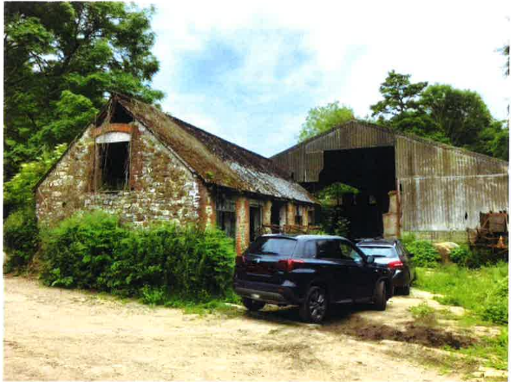
Building C: Single storey construction with rendered masonry external walls and corrugated cement based sheets supported on steel trusses.
