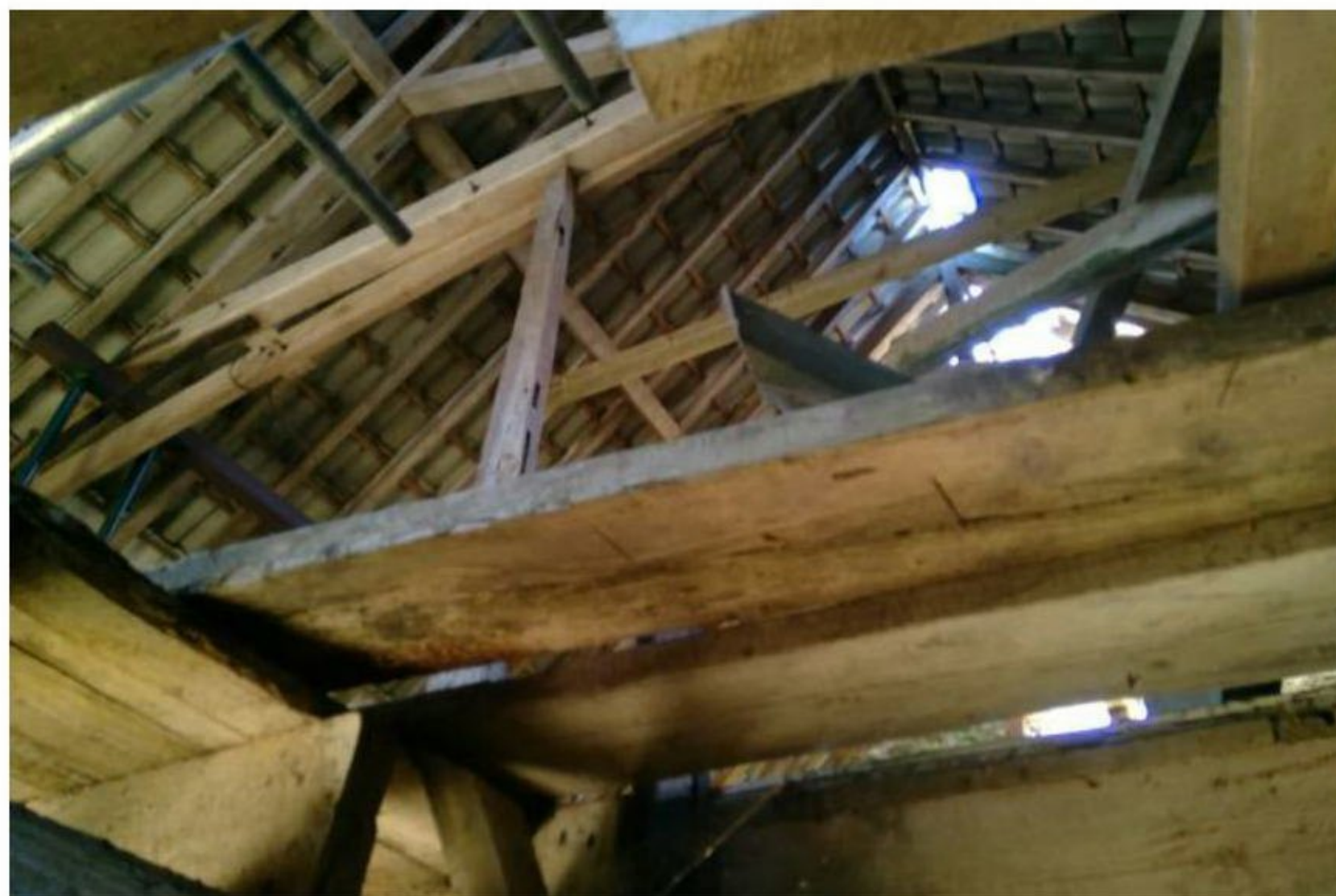
Photo 2: interior of Building A showing gap in ground floor ceiling to first floor and roof.
