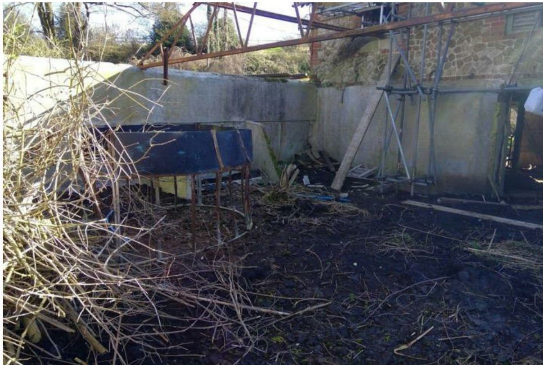
Phot 6: Interior of Building C showing missing roof.
