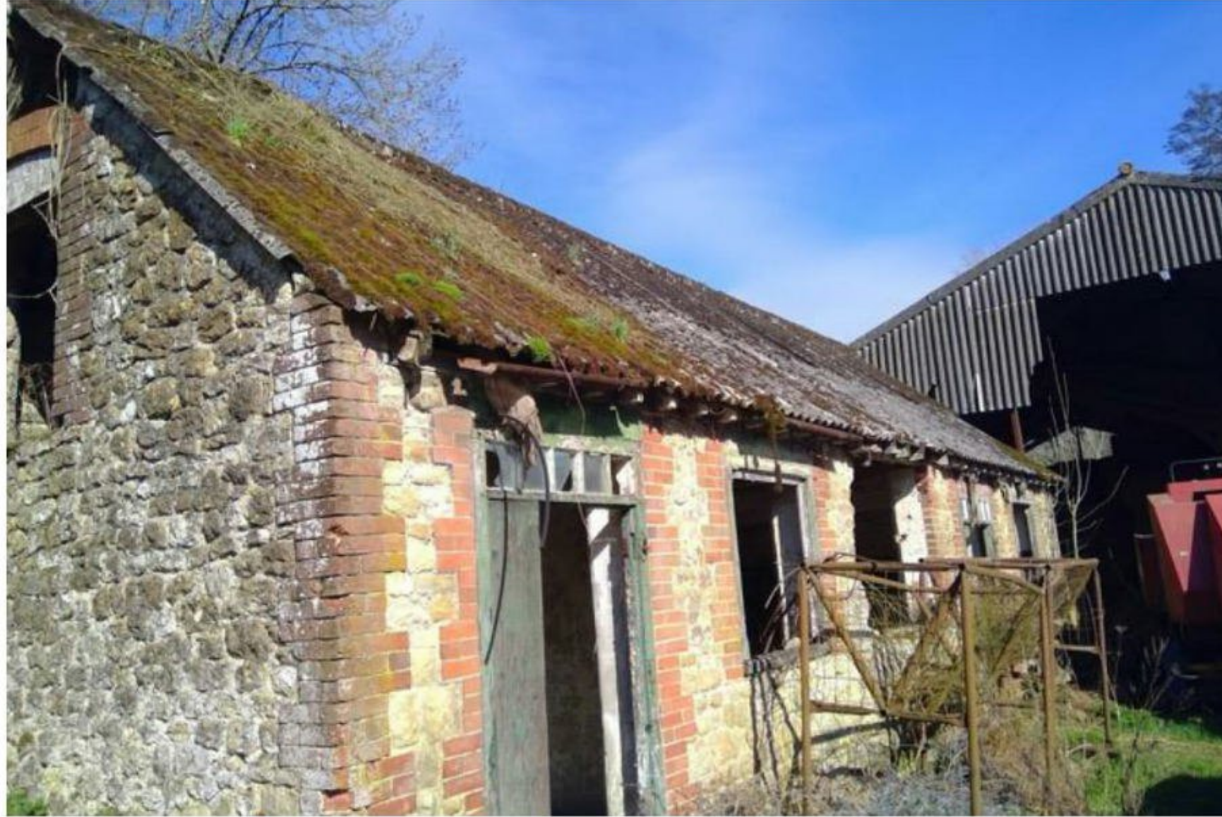
Photo 3: Showing exterior of Building B with potential entry points.
