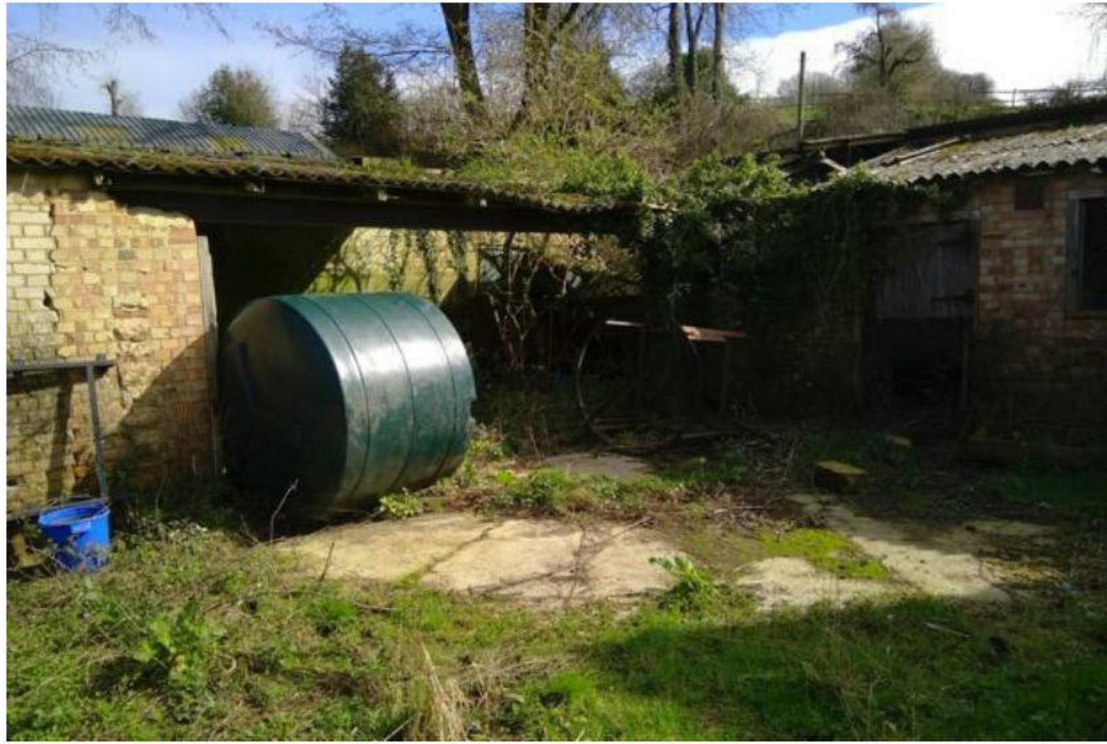
Photo 7: Exterior of Building D showing potential access points and tree growing in corner section.
