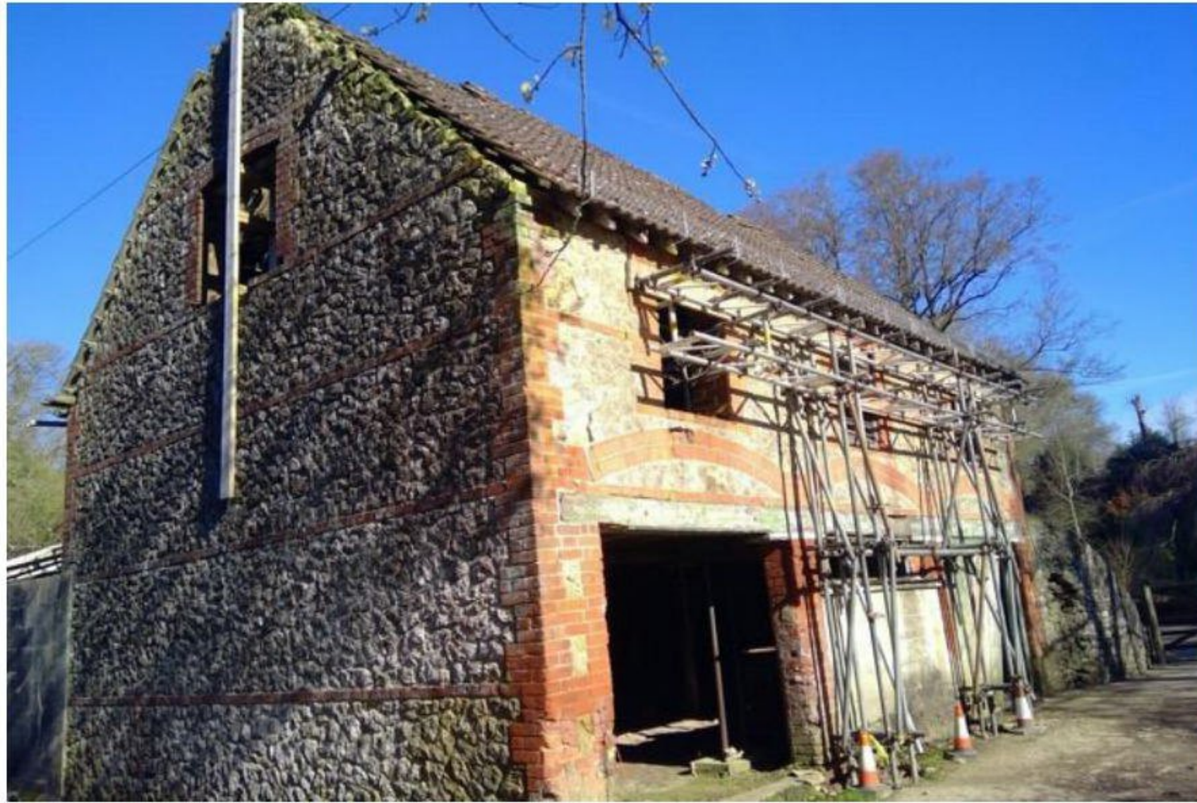
Photo 1: Building A. Showing possible entry points in roof and windows.
