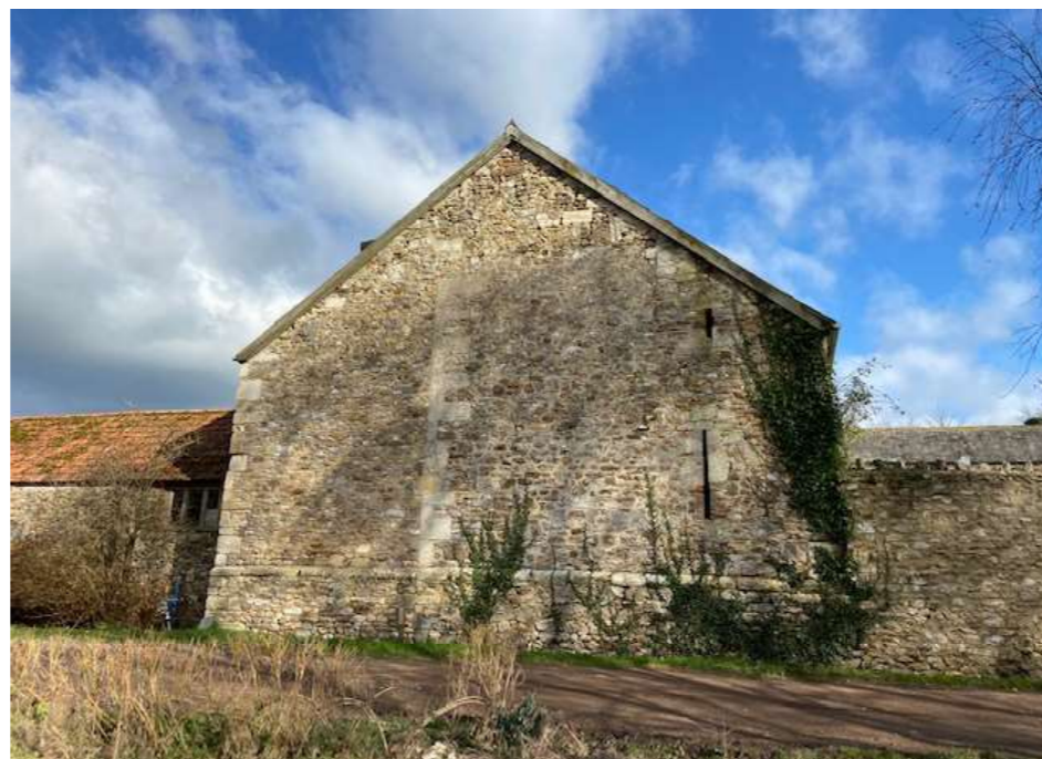
Fig 20. West elevation of Manor Barn showing quoins mid way along wall where earlier building has been extended.
