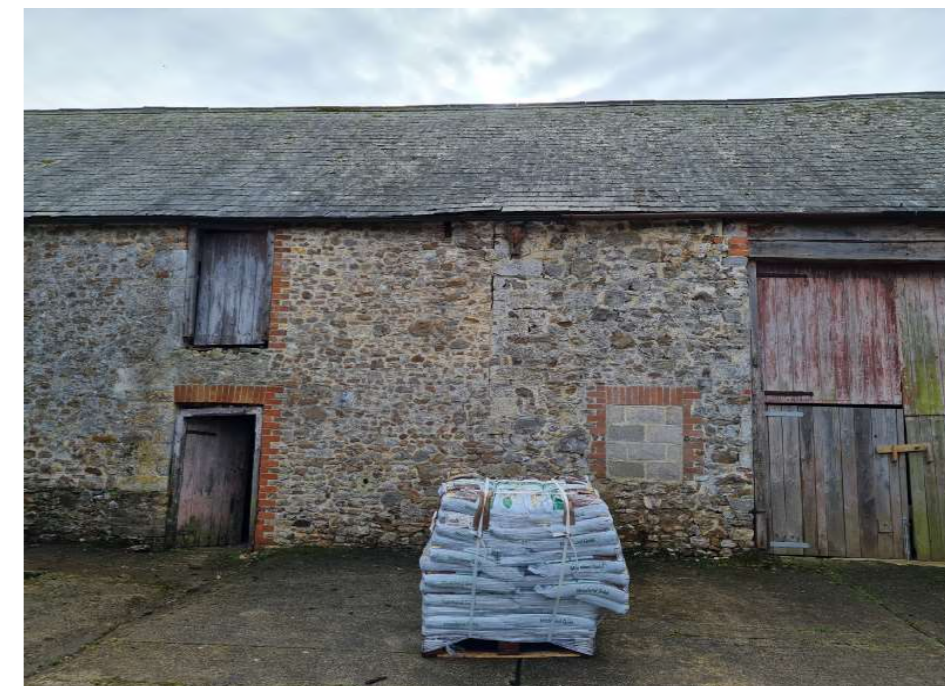
Fig 21. North elevation of Manor Barn showing quoins mid way along wall where earlier building has been extended.
