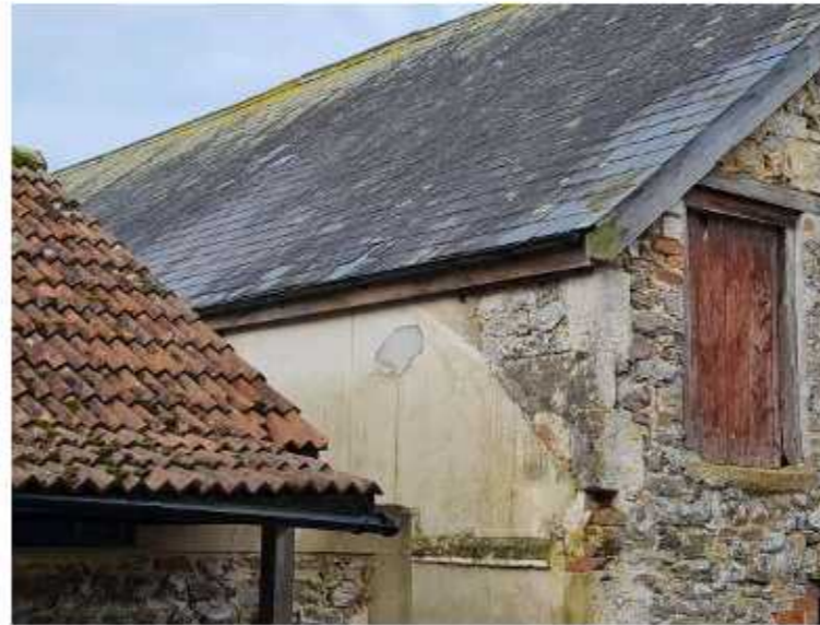
Fig 17. Photo showing 'tide mark' of former roof of dairy barn connecting with the manor barn.
