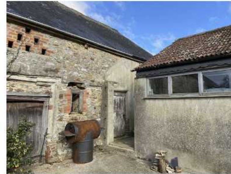
Fig 18. Photo showing 'tide mark' of former roof of dairy barn connecting with the manor barn as viewed from southern courtyard.
