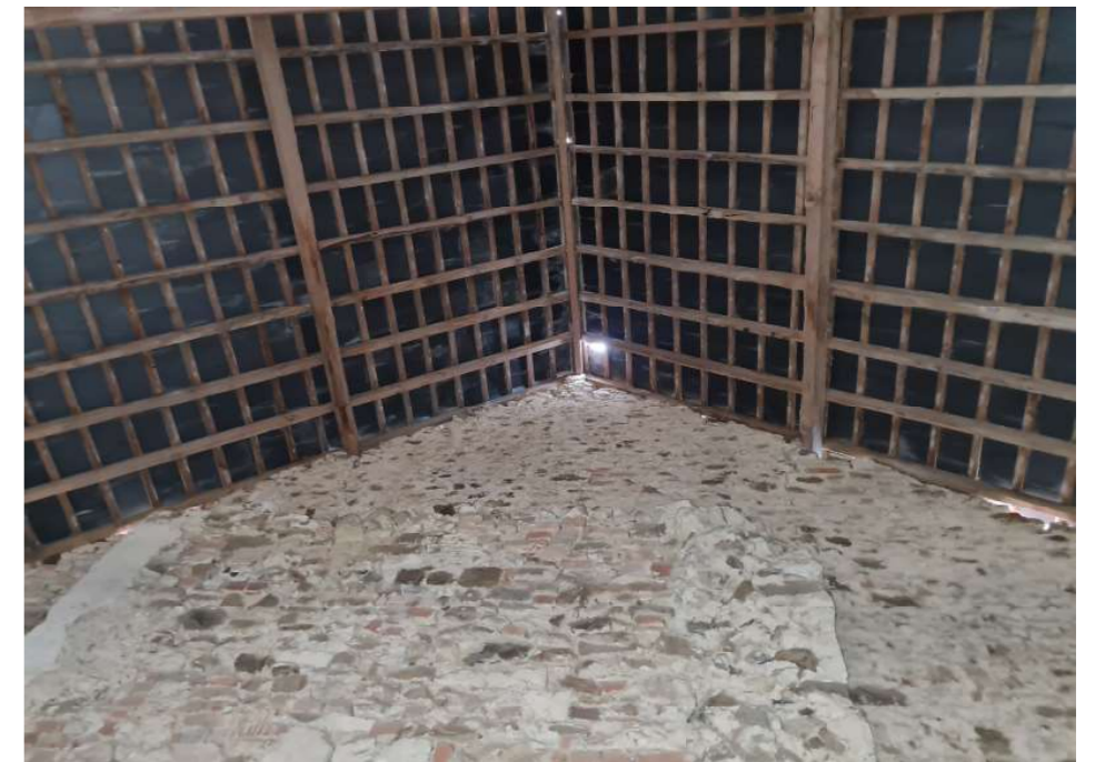
Fig 16. Detail photograph of internal side of western gable of barn looking up to roof.
