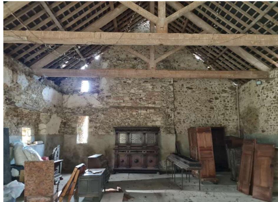
Fig 13. Existing barn looking west towards western gable and location of proposed reinstated fireplace.
