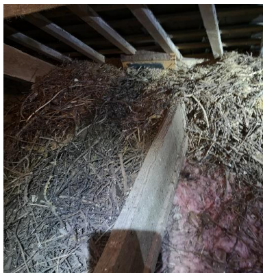
Figure 8. A corvid nest within the loft void of the Farmhouse
