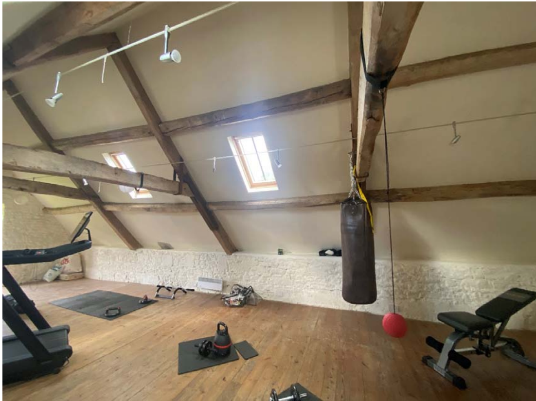
Figure 5: Location of roof trusses has informed the proposed rooflight design and position
