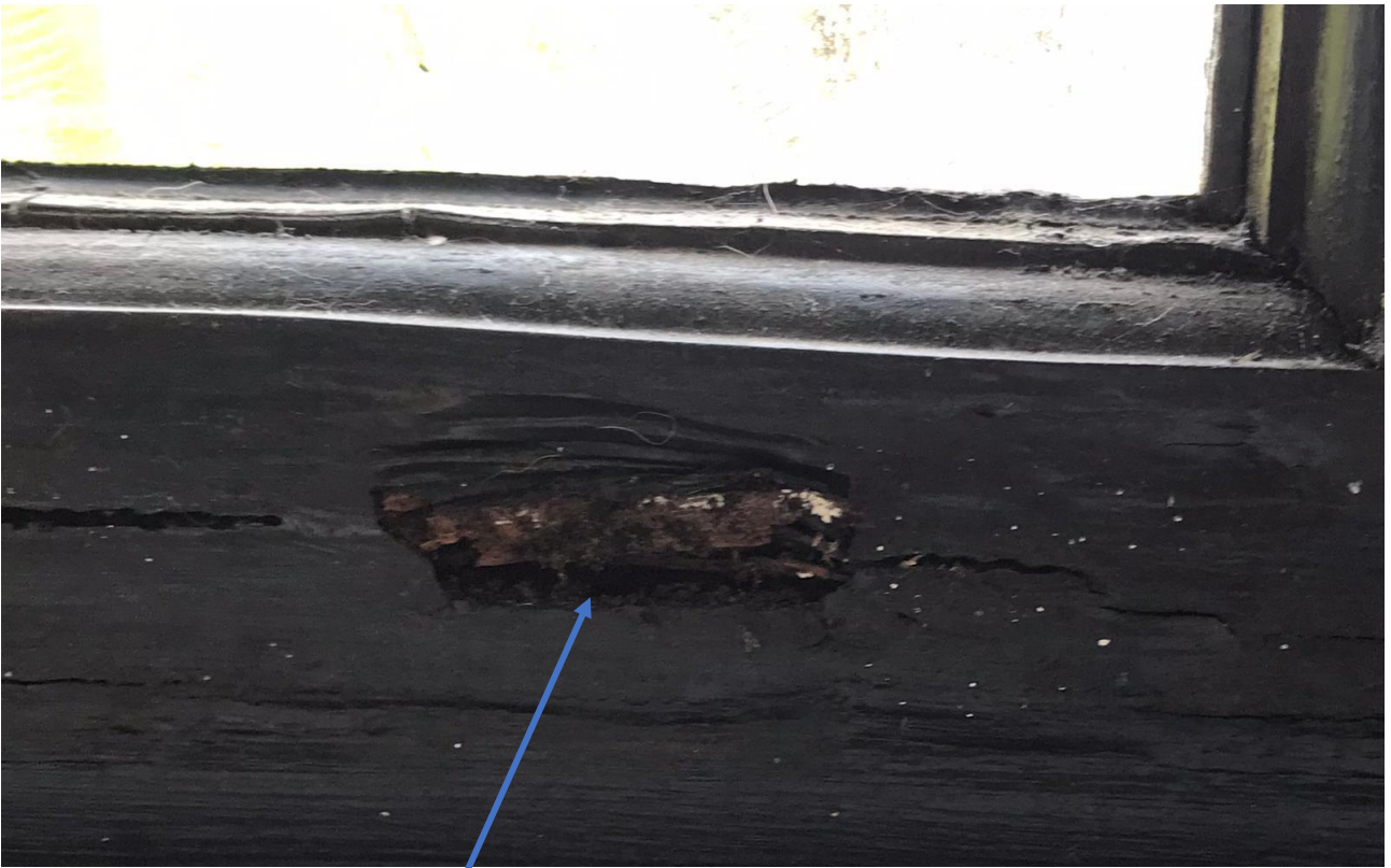
Internal window 1 - Rotten wood and covered by black paint
