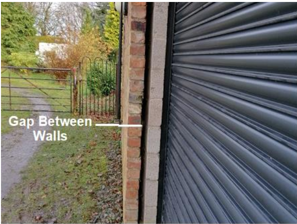
PHOTO 7 View of Wall Cavity Gap
