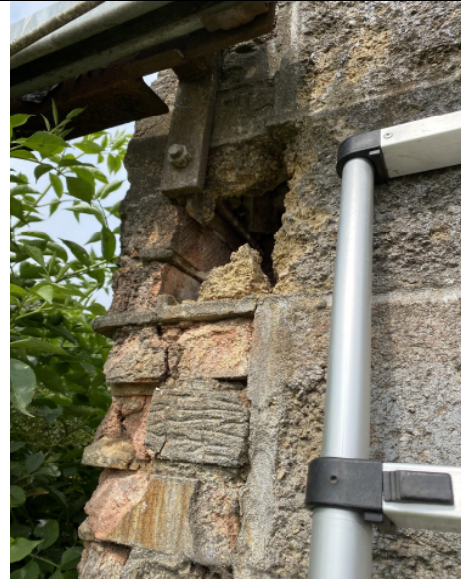
Close up of largest crevice (TN1)
