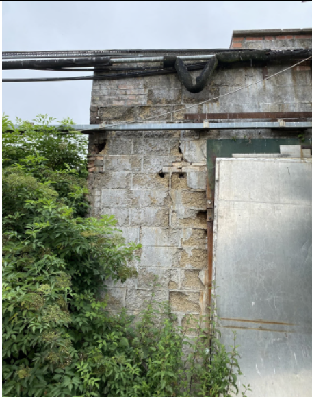
Wall between Structure S1a and S1b showing multiple crevices due to deteriorating construction materials (TN1)
