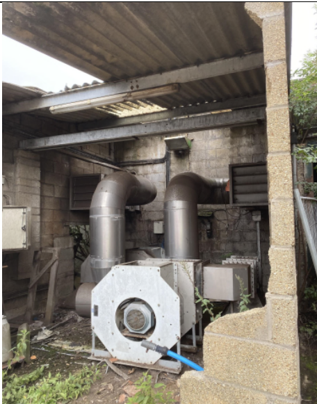
General view of Structure S1a showing poor state of repair and abandoned ventilation equipment
