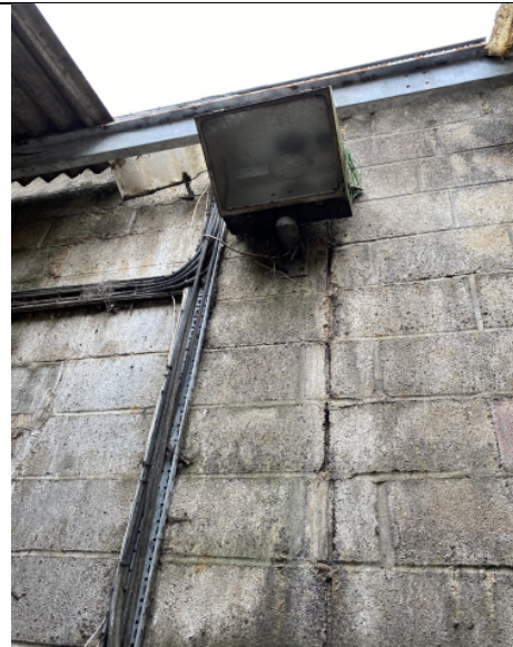
Open roof of Structure S1a due to missing roof panels and remanent of pigeon nest (TN3)
