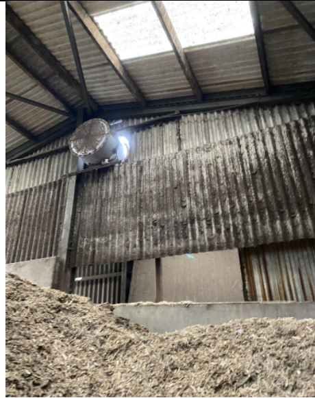
Far end of Structure 2 showing wood pulp pile and damaged interior wall
