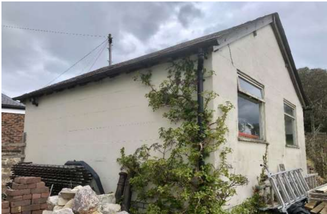
Fig 8: The existing garage is a modern building built of concrete breeze-blocks, metal casement windows and a timber framed roof. It is of no significance to the setting of the listed building and can be replaced.
