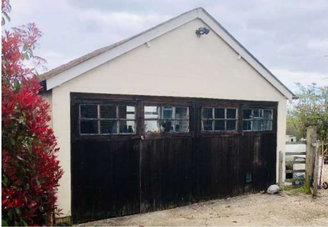
Fig 7: The existing garage consists of a building built of concrete breeze-blocks and dates from the late 20 th Century. Although the front timber doors appear traditional, they have been previously recycled.
