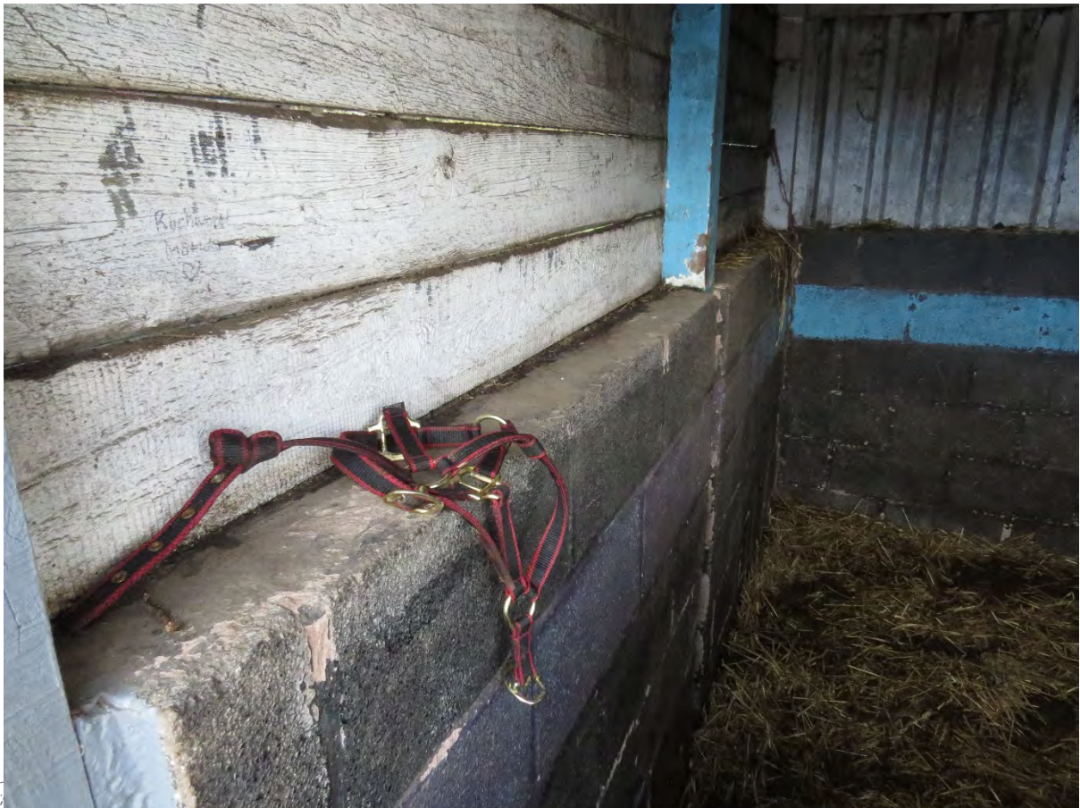
6 – Base walls are solid blockwork or brickwork, with single layer timber or sheet metal walls.
