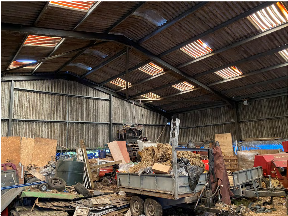
4 – Internally the walls are not lined and there are no features suitable for use by roosting bats.
