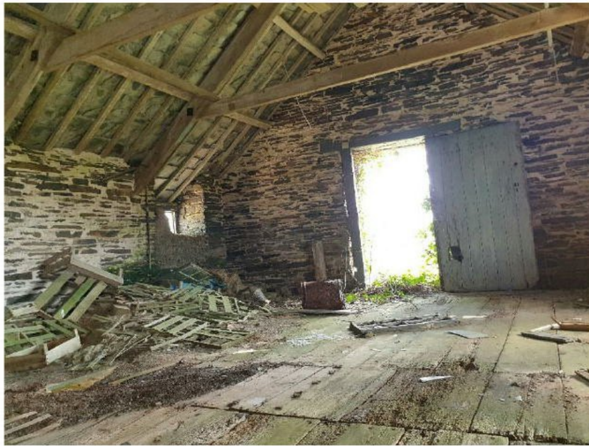
Figure 18: Interior of first floor of two-storey section of Barn 2 at Porthmissen Farm (viewed towards the east)
