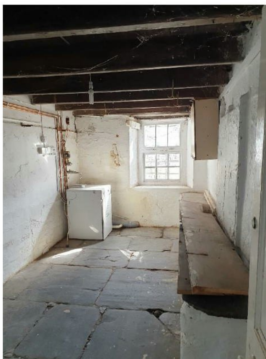
Figure 5: Interior of one of the ground floor rooms within the farmhouse at Porthmissen Farm
