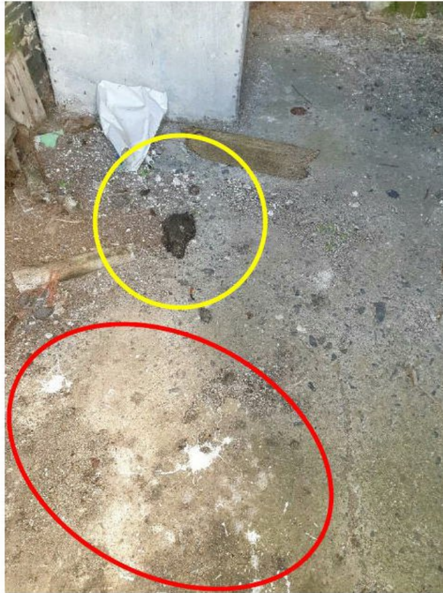
Figure 24: Barn owl pellet (yellow circle) and liming (red circle) on floor of the single-storey section of Barn 1 at Porthmissen Farm
