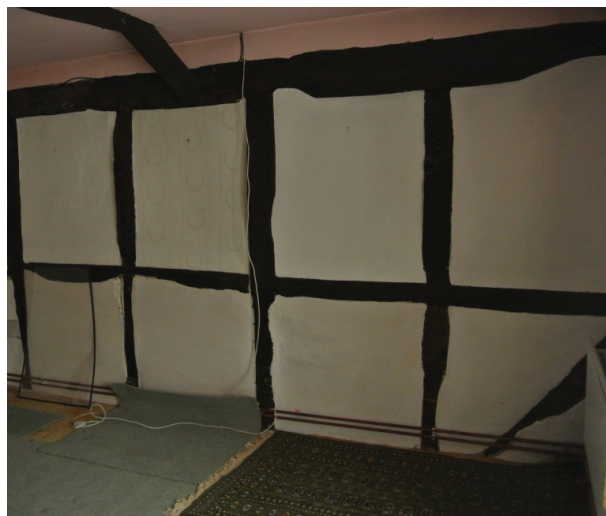
Fig 2.18 Bedroom 1 pipework to be rerouted within existing floor service void. All existing redundant cabling stripped out and plaster to be repaired
