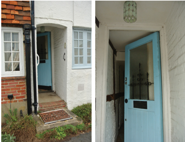
Fig 2.13 Front door to be redecorated, step at front to be repaired
