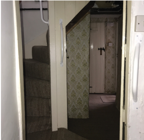
Fig 2.10 Dark stairwell with steep staircase case and step 1 plinth
