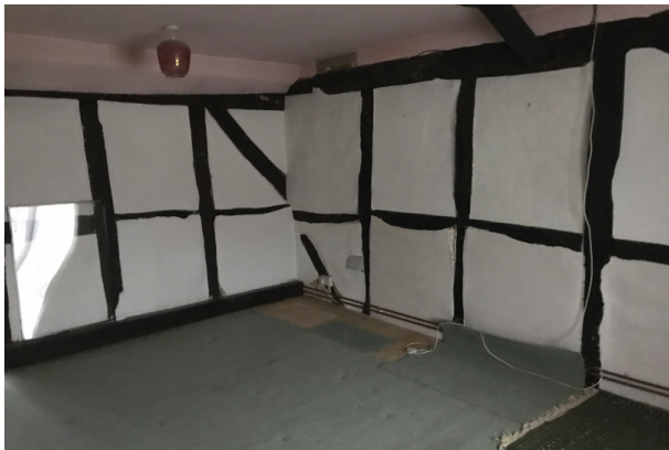
Fig 2.15 Bedroom 1 corner proposed en-suite location. Low level boxing on left (painted brown) which conceals pipework is to be removed and radiator pipework rerouted in existing raised floor void.
