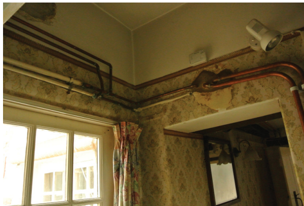
Fig 2.16 Pipework in existing rear lobby by boiler to be removed and rerouted to conceal it. Opening on right to be widened towards the left and door to be moved further out.
