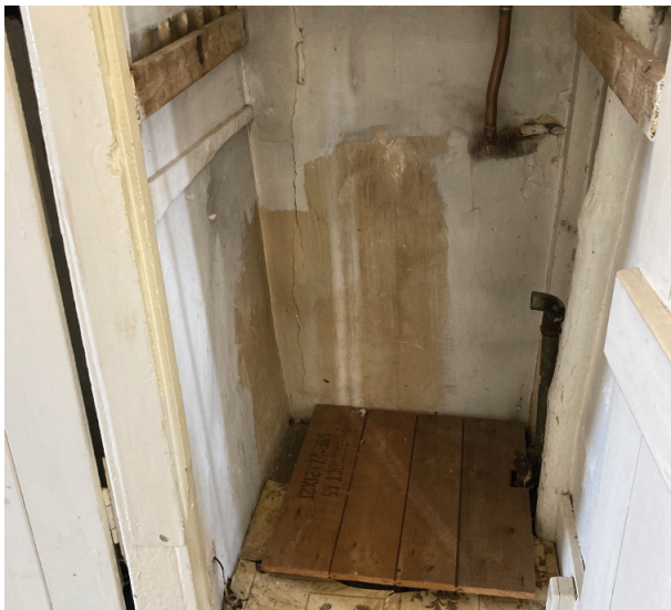
Fig 2.12: 1970's landing cupboard which impinges on head height over stairs and has remnants of old plumbing
