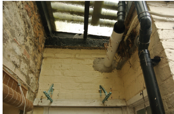
Fig 2.3 Polycarbonate roof to rear extensions, (rear wall of the historic house on the left. Boiler flue and pipework to be removed)
