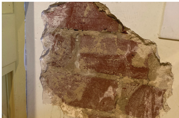
Fig 2.2 Modern oddly constructed 1/4 brick wall between existing hall and kitchen to be removed
