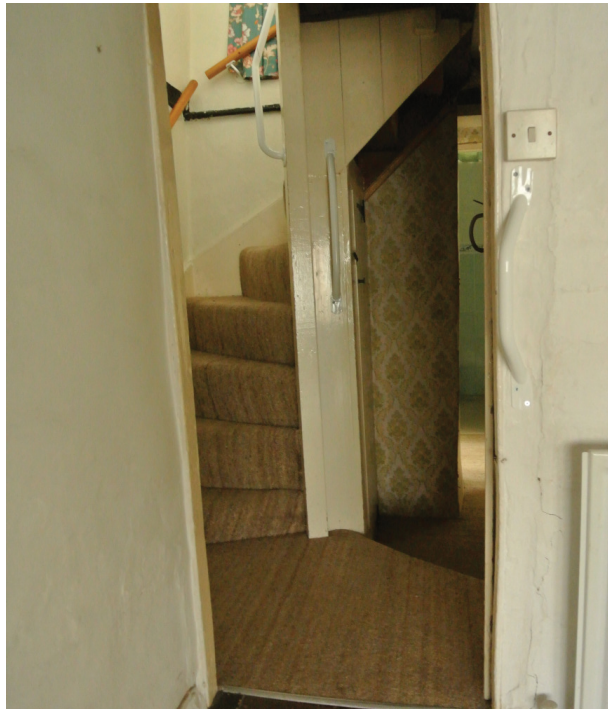
Fig 2.1 Staircase with steep pitch and step 1 plinth
